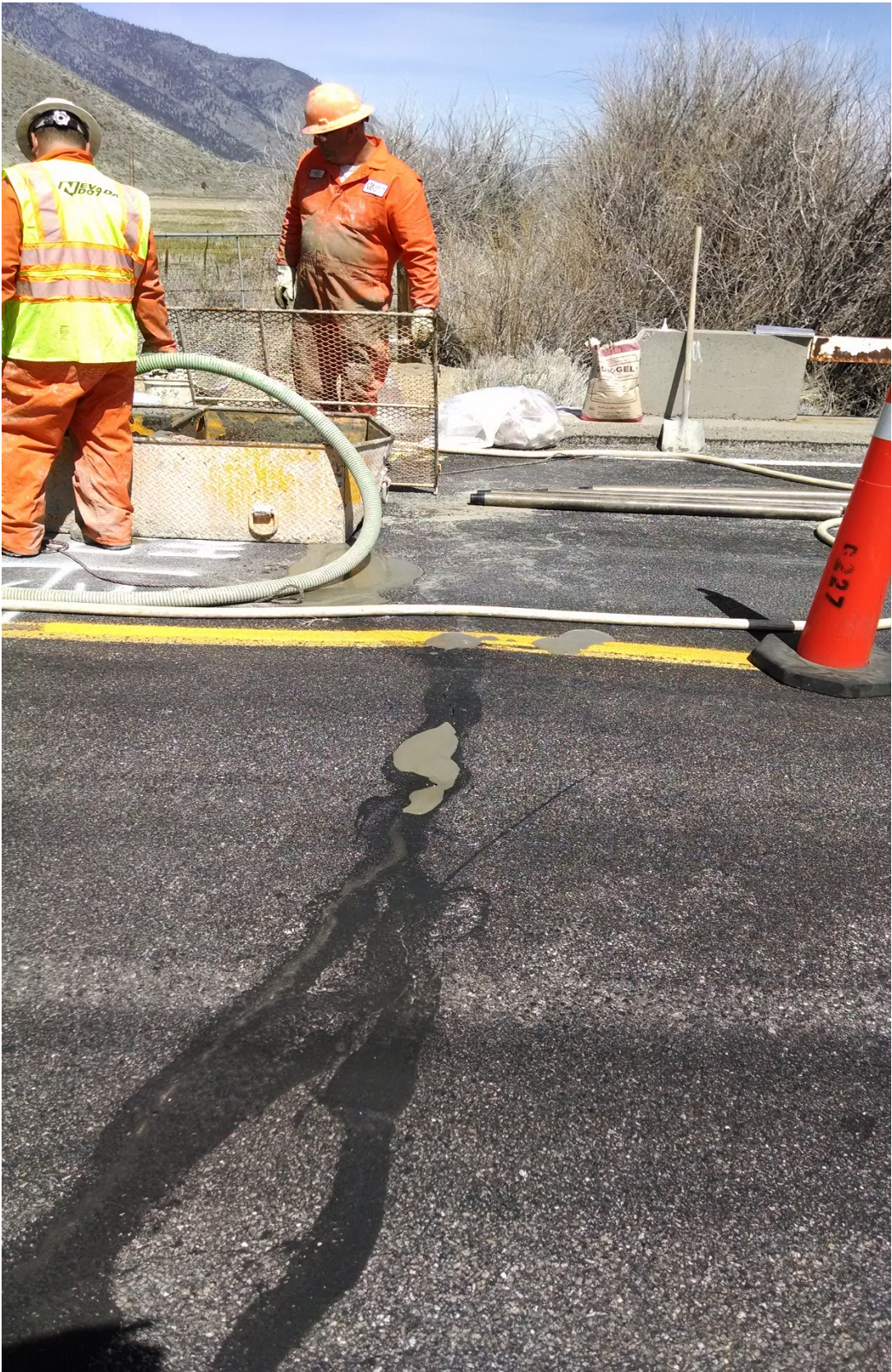
Pavement distress and drilling fluid upwelling through pavement at Borehole MU-1
