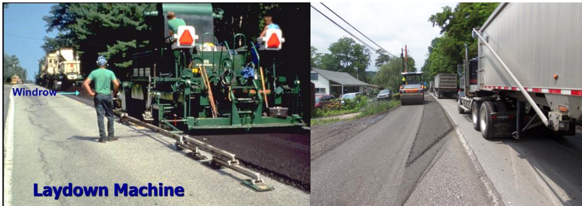
Figure 2. The CIR mix is picked up by the paver and roller compacted.
