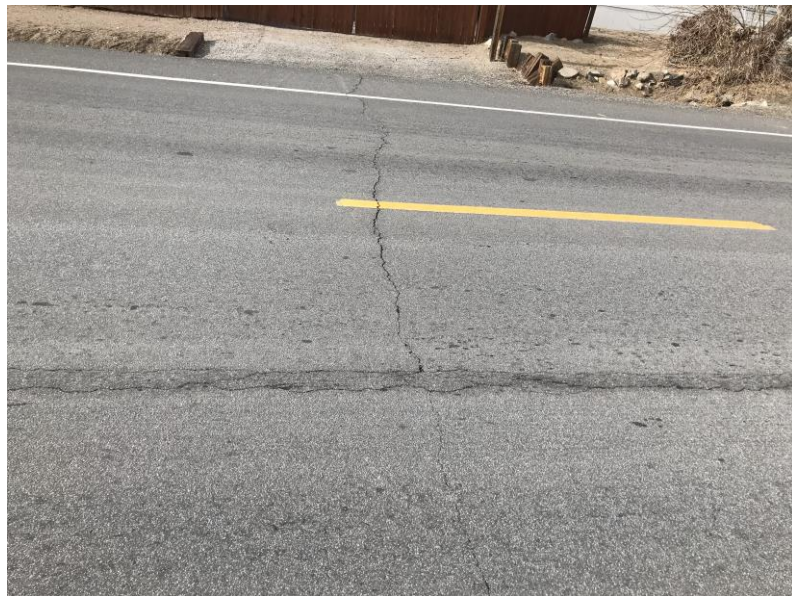
Figure 4. Surface of Sandpiper Drive in December 2017.
