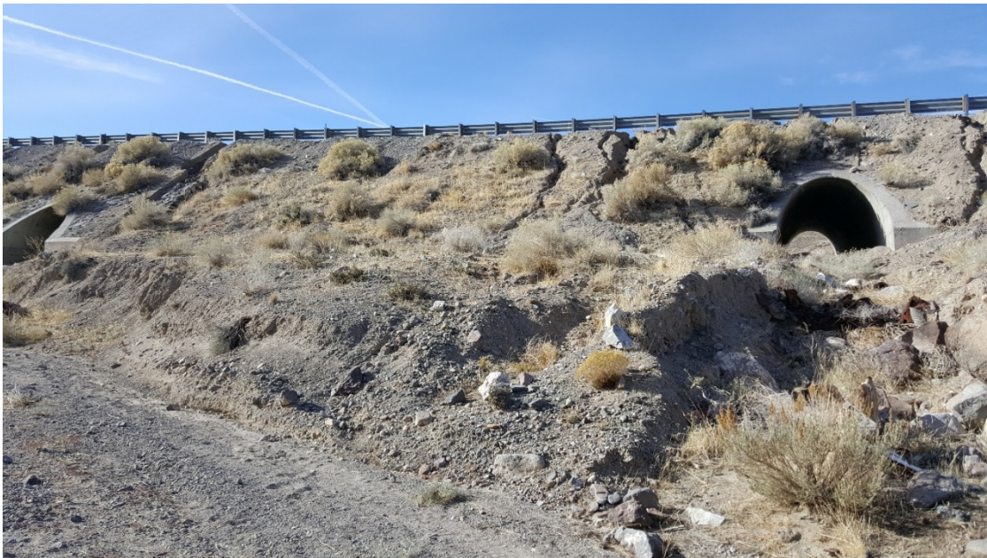
Northern barrel of double concrete arch box (left) and single barrel concrete arch box (right). Photo looking west.
