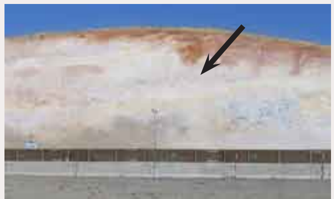
(3) Not Recommended: Flat, Uncontoured Cut Slopes of 2H:1V. • Reduces likelihood of successful revegetation on steep slope. • Appears dull and stark against the contextual landscape.
