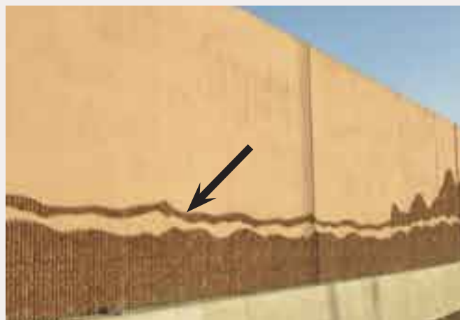
(1) Not Recommended: Disproportionately Applying Relief Pattern – Pattern Applied too Low on Wall.
