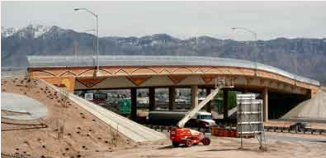
(1) In this example, color and pattern have been applied to decorate the bridge after the design decisions have been made. The result does not necessarily create an aesthetic structure. The point is that applying decoration does not necessarily make it more appealing.
