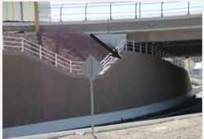
(2) Not Recommended: Tall Retaining Walls Directly Parallel Travel Lanes.
