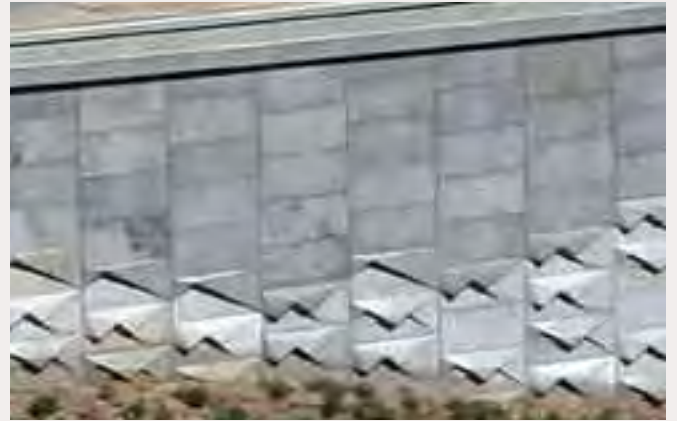
(1) Panel size and shape have direct bearing on aesthetic composition. Larger panels such as those shown above tend to reduce the visual impact of numerous joint lines.
