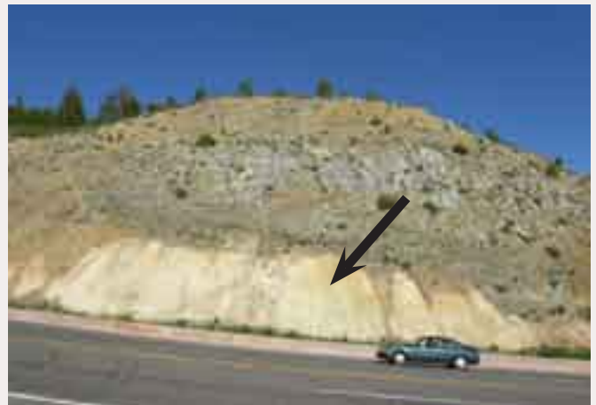
(2) Not Recommended: Unstained Cut Slopes. • Draws additional attention to cut slope because of contrasting color with lightly colored cut slope.
