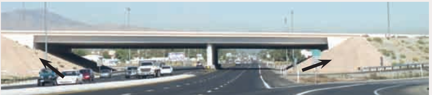
(3) Not Recommended: Paved Embankment Slopes.
