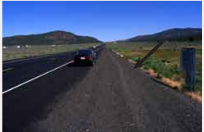
(1) Not Recommended: Roadway Millings Used for Shouldering Material.
