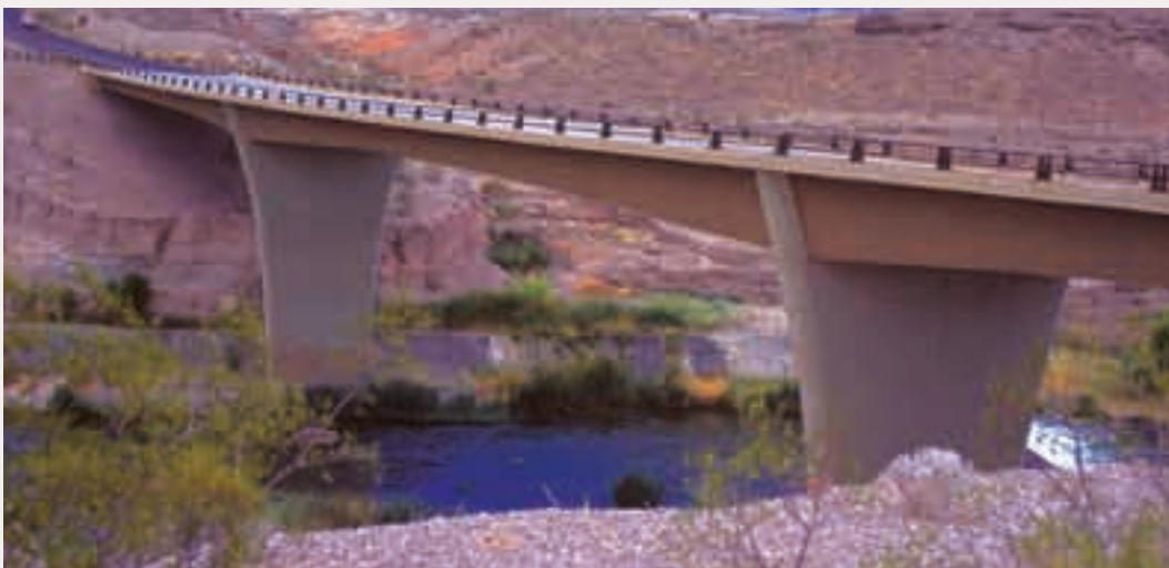
(2) This structure's graceful form and composition indicate that the aesthetics of all its features were considered together during preliminary design. The fact the structure blends with the environment is appealing.
