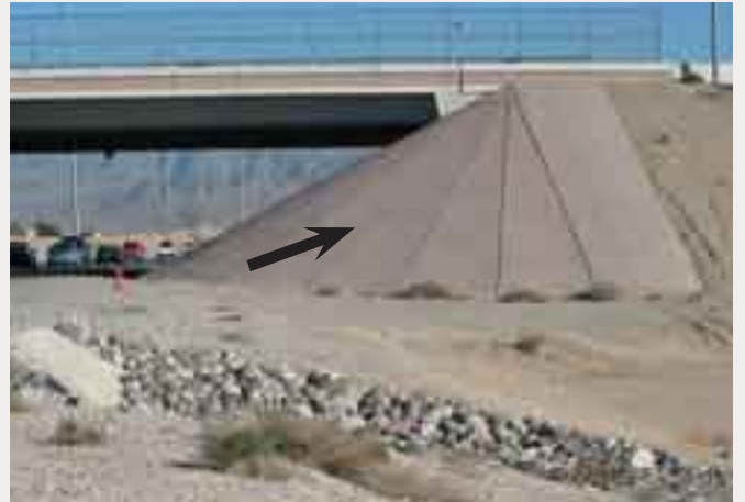
(1) Not Recommended: Paved Embankment Slopes.
