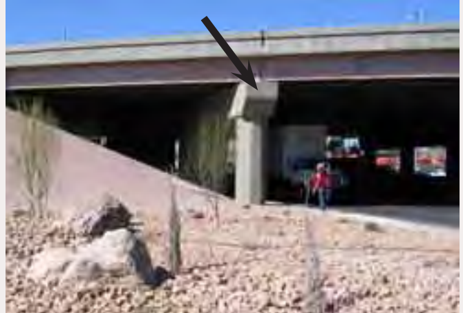
(1) Not Recommended: Exposed Pier Cap.
