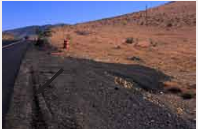
(2) Not Recommended: Roadway Millings Used for Shouldering Material.
