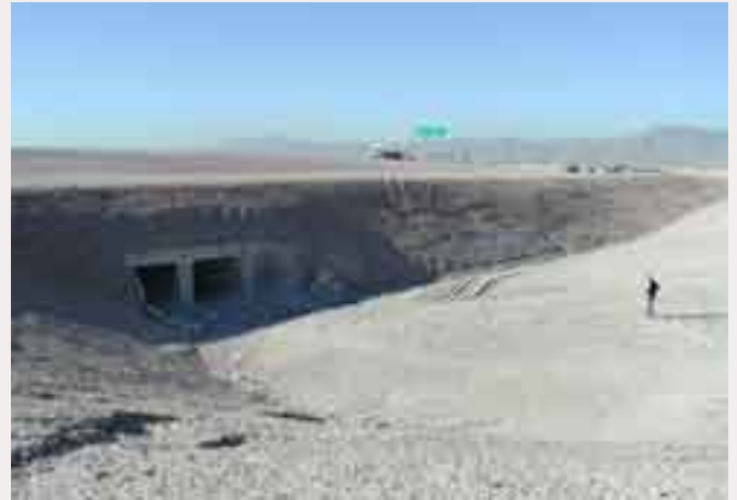
(1) Drainage facilities can be a visually dominating feature because of the scale needed to handle flows. The facility shown above requires aesthetic design consideration to try and blend it into the natural landscape so it does not create an eyesore.
