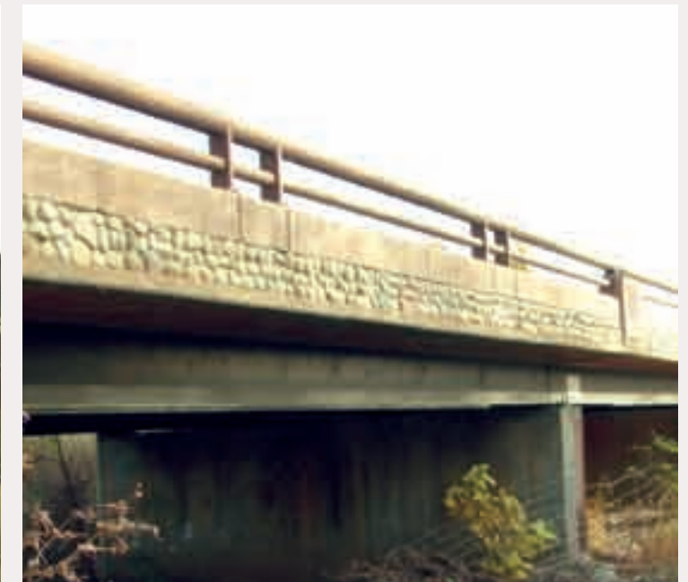
(13) Bridges should be uncomplicated. Open rails create a more refined appearance and maintain views.
