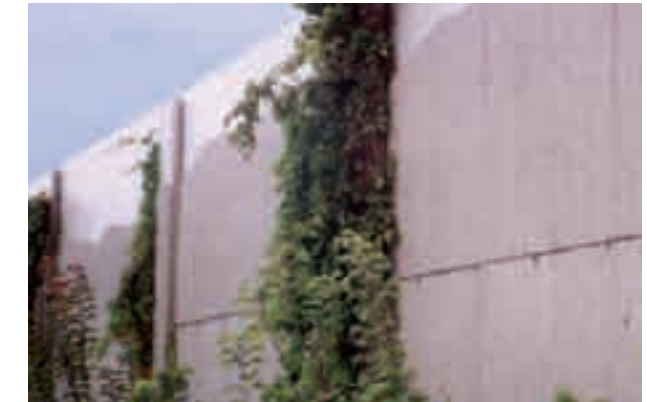
(7) The integration of vertical vegetation softens noise walls.
