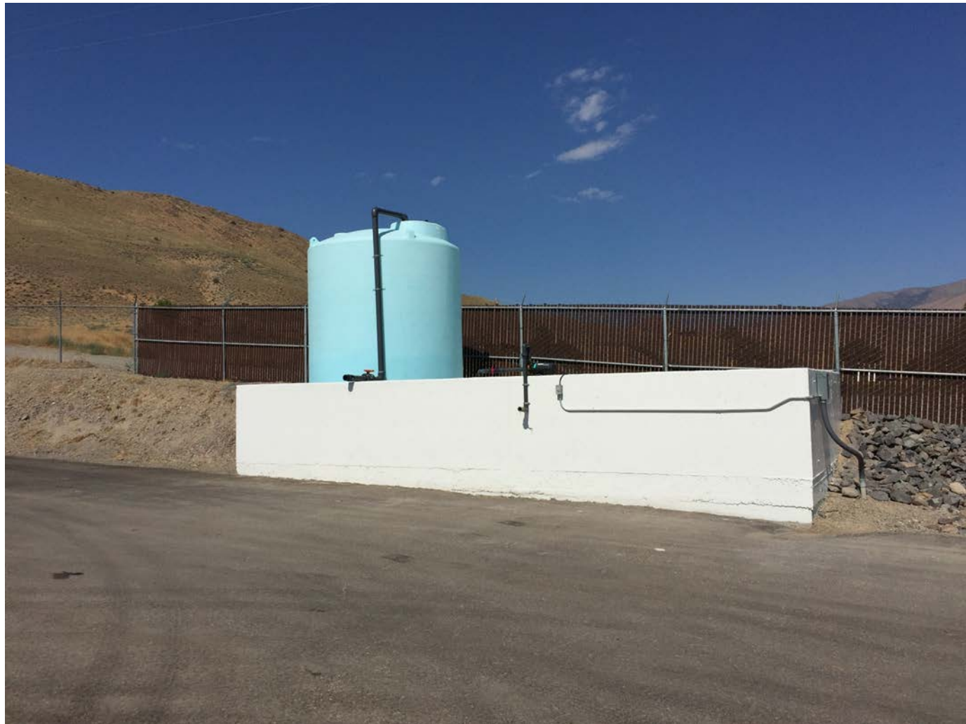
Brine tank secondary containment structure (Wellington Station)
