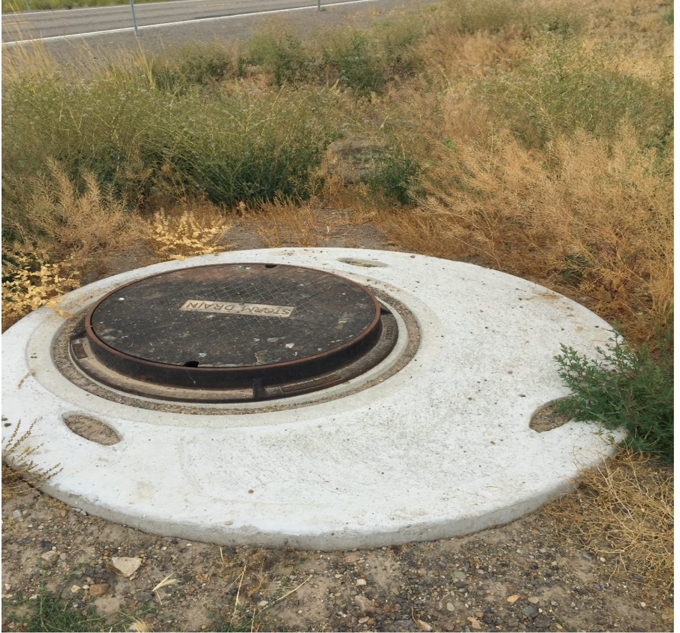
Stormwater treatment vault (North Fork Station)
