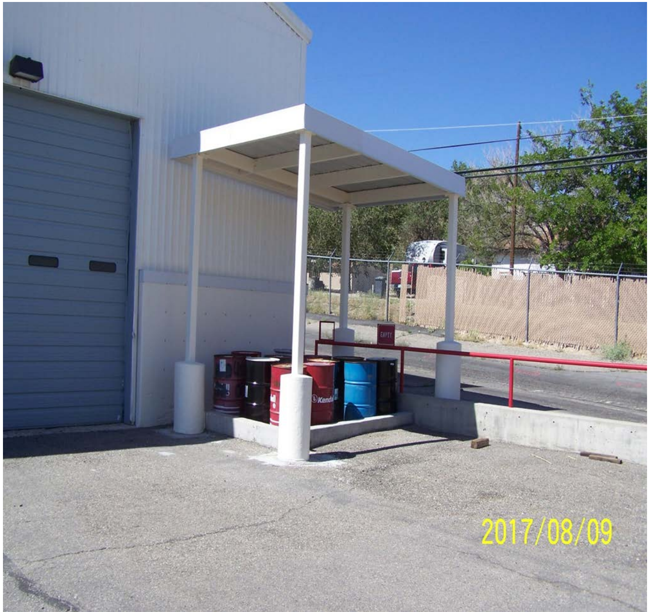
Outdoor materials storage area overhead cover and secondary containment (Tonopah Station)
