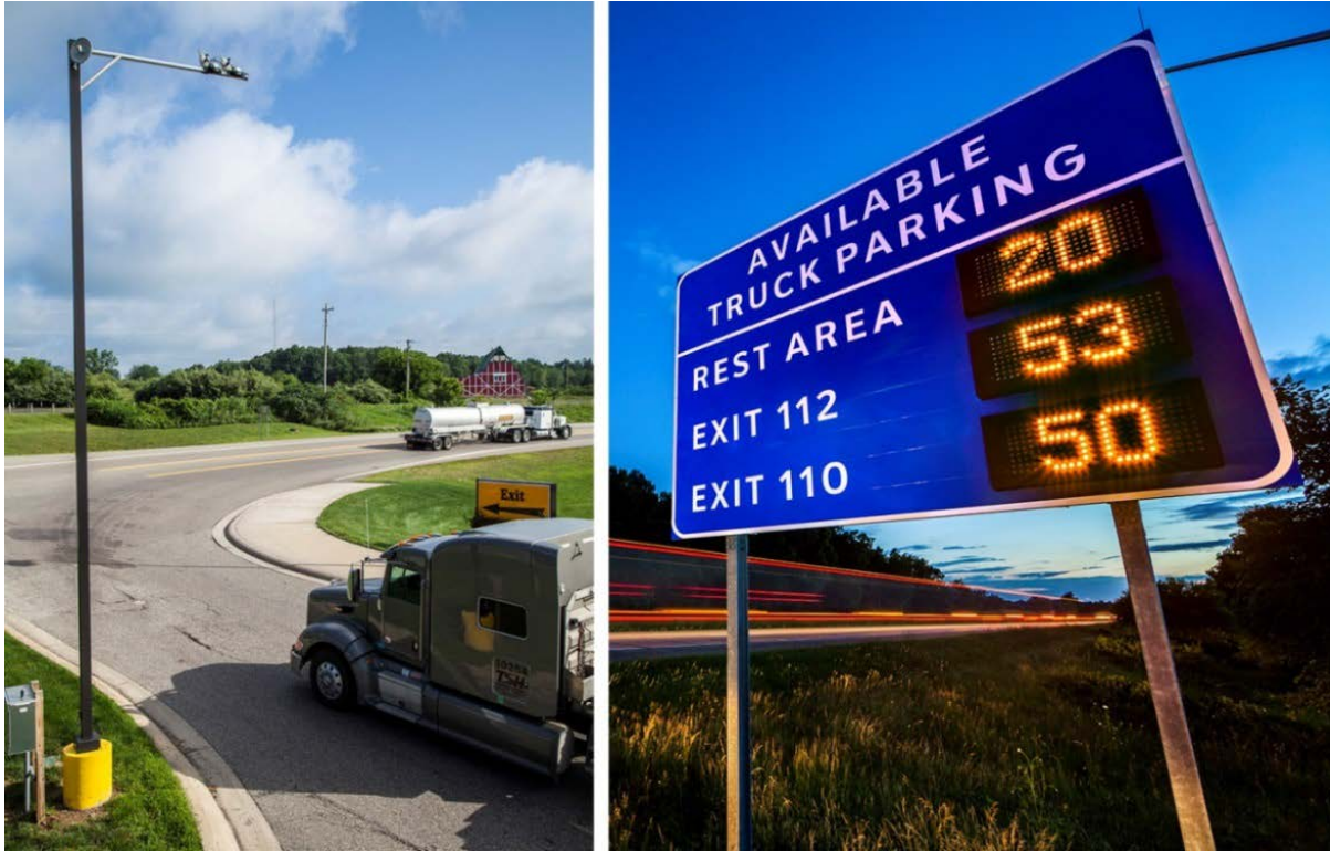
Figure 8.5 TPIMS Monitoring Equipment (left) and Dynamic Real-Time Message Sign (right)
