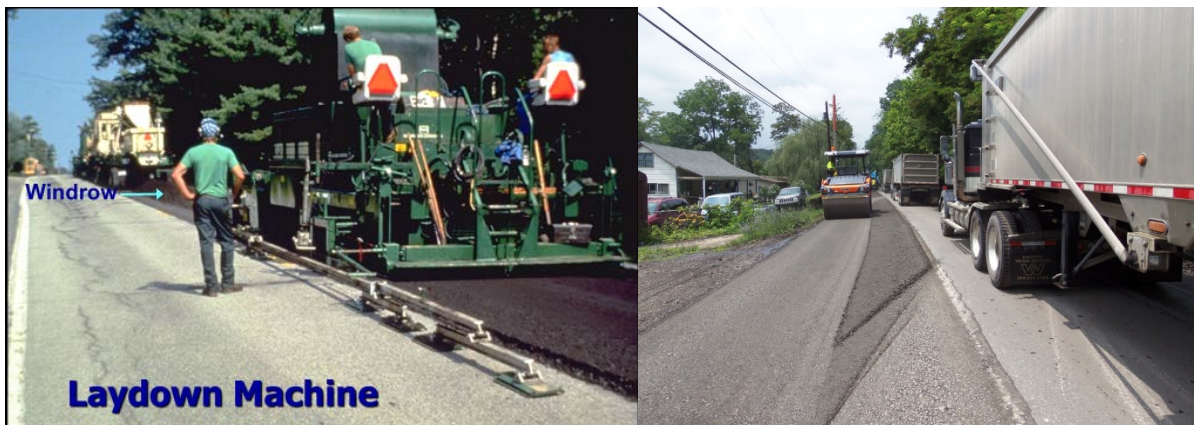
Figure 1.2. The CIR mix is picked up by the paver and roller compacted.
