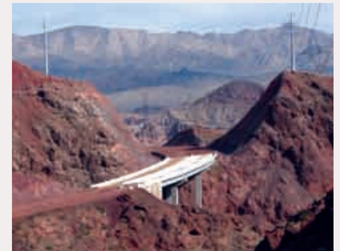
(1) New bypass construction near Hoover Dam and Lake Mead is an opportunity to provide enhanced roadside services such as a welcome center and safe viewpoint pull-offs.
