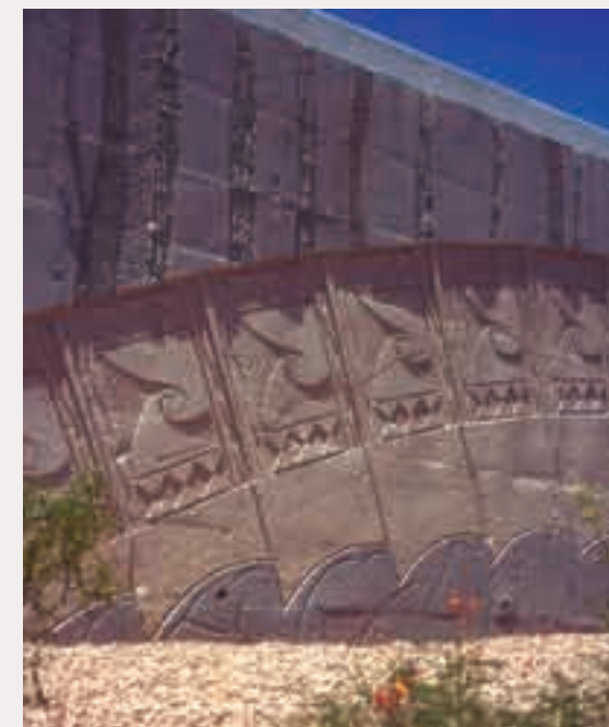
(2) Decorative imprint motifs can be created with a custom form liner and used to decorate walls.
