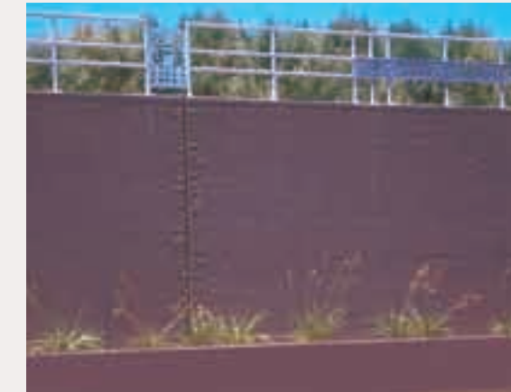
(2) Retaining and noise walls should be separated from concrete barriers and other structures to allow space for landscape planting.
