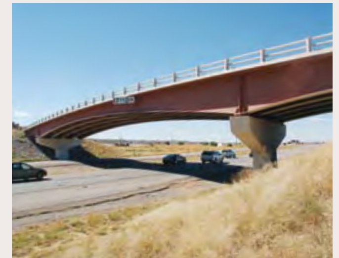
(2) Simple color application as part of a retrofit project can improve the aesthetic quality of existing bridges and structures.
