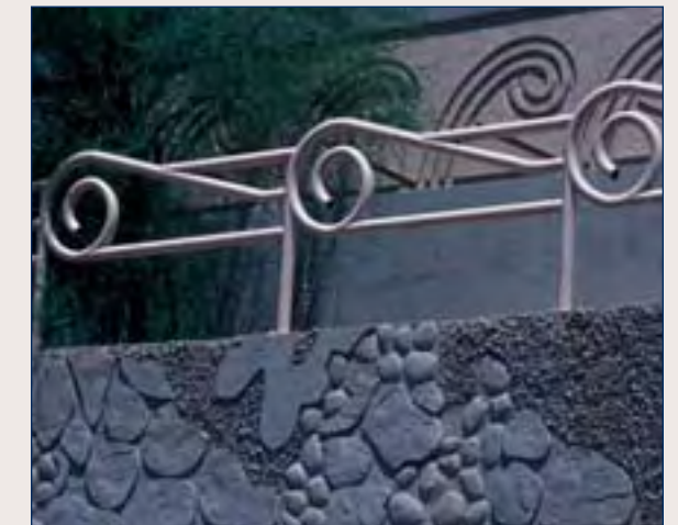
(6) Retaining wall and pedestrian walkway with desert visual design theme created with concrete form liners.
