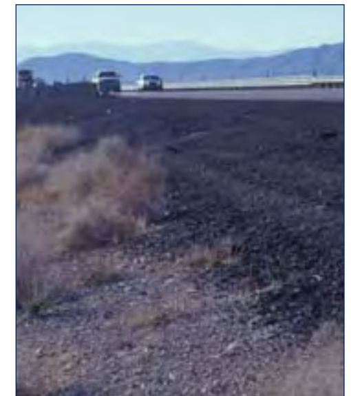
(4) Existing condition of asphalt millings being placed along the shoulder should be reused in repaving projects.
