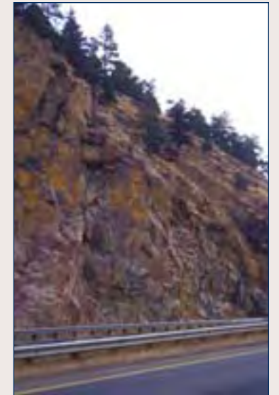
(5) Example of the rock cut in which natural bedding planes were used to excavate naturalized landform. Weathering techniques blend this rock cut.
