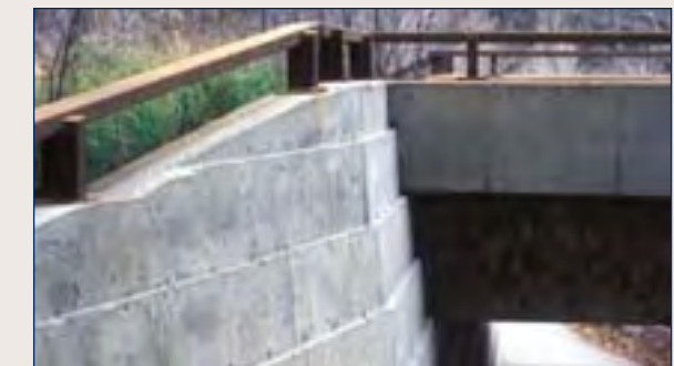
(9) Pedestrian underpass integrated into highway bridge design, rather than separate structure design. Height of opening allows light into underpass.
