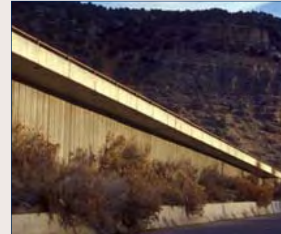
(2) An example of a cantilevered retaining wall with a simple, consistent use of materials. Vertical joints are most compatible with the finish.
