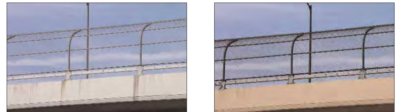
(4) The following images demonstrate existing roadway structures before and after color palette application. Color application can be retrofitted to existing-in-place structures.
