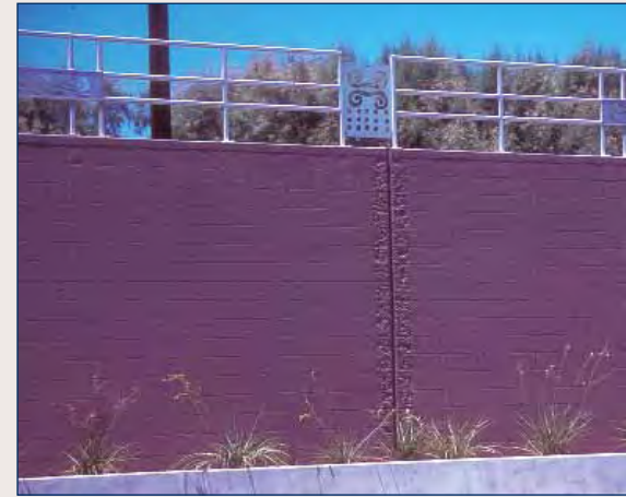
(5) Simple retaining wall pattering, railing design, and landscape palette. The wall is separated from the concrete barrier with the space and planting area.
