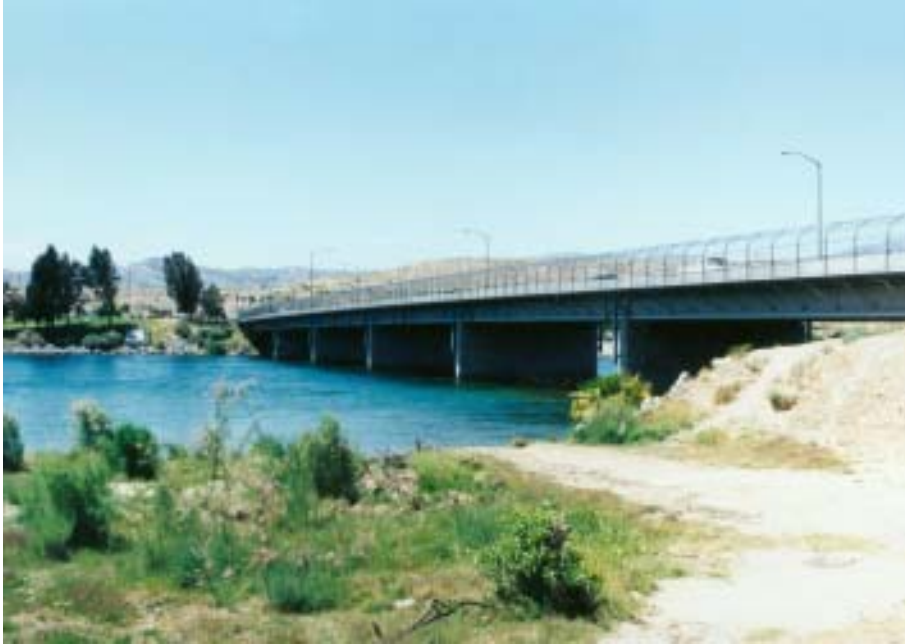
US 95 bridge over the Colorado River, looking west from Bullhead City, Arizona, to Laughlin, Nevada.
