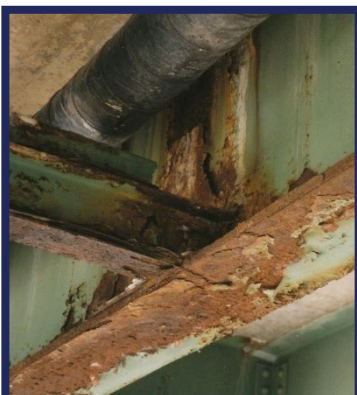
Figure 4-4. Example of deteriorated steel on a bridge girder.
