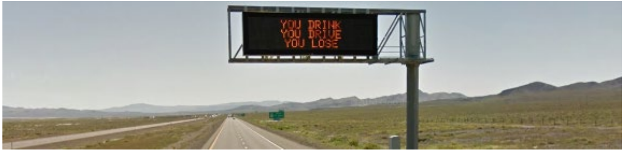
Figure 5.1 Dynamic Message Sign (I-80 westbound) Near Exit 83 (Fallon)
