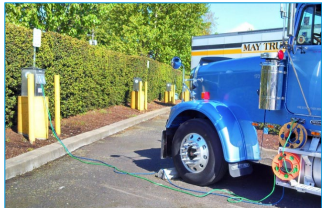
Truck Stop Electrification
