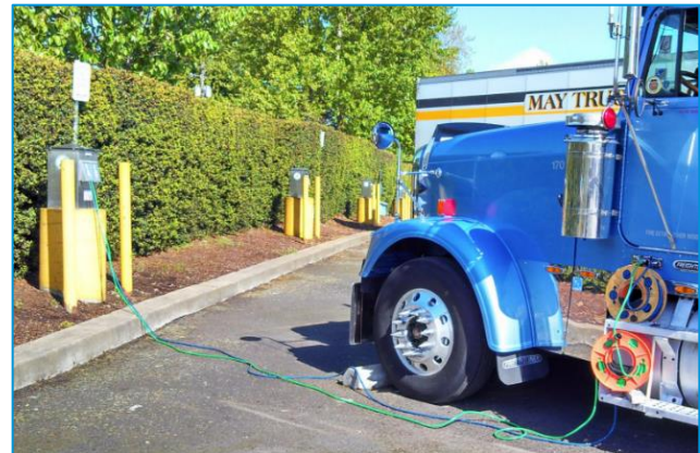
Truck Stop Electrification
