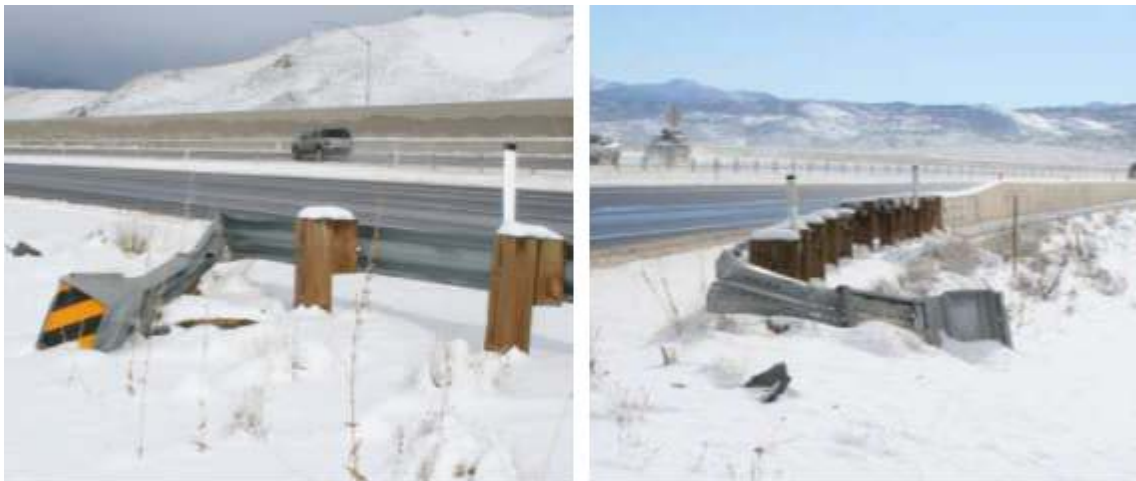
Deficient Impact Attenuator/ End Treatment:
