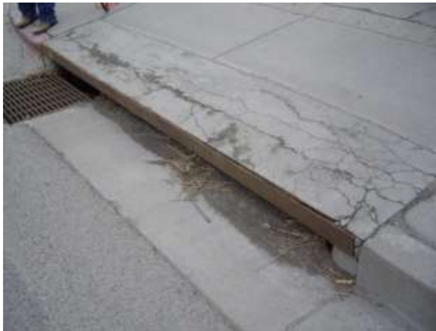
Deficient Drop Inlet:
