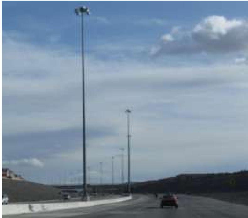
Example of Highway Lighting (High Mast Lights):
