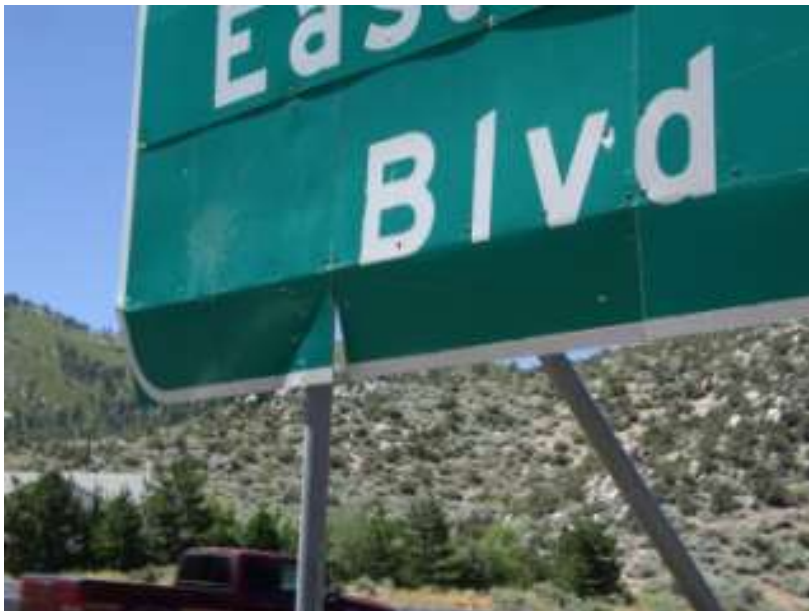
Damaged Traffic Sign:
