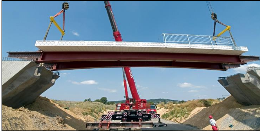
Figure 6: A 21.5 m FRP deck placed on top of steel girders to create a traffic bridge over B3 highway in Germany [50].
