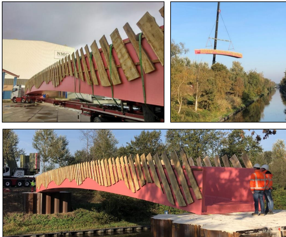
Figure 10: Installation of a uni-mold FRP ecoduct near Eindhoven, The Netherlands. Bridge is 36m x 3.5m [63]. Top left; bridge is delivered in one piece from the factory to the construction site. Top right; bridge is lifted into place using one crane. Bottom; FRP ecoduct is placed onto abutments over a canal.
