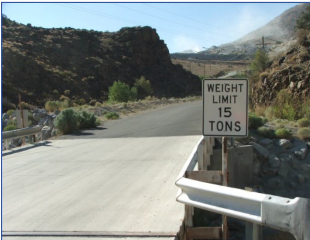
Example of Structurally Deficient Bridge
