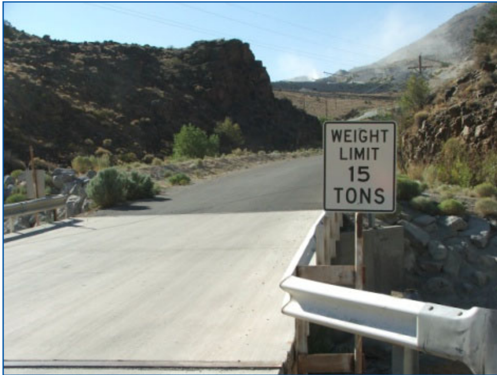
Example of Structurally Deficient Bridge
