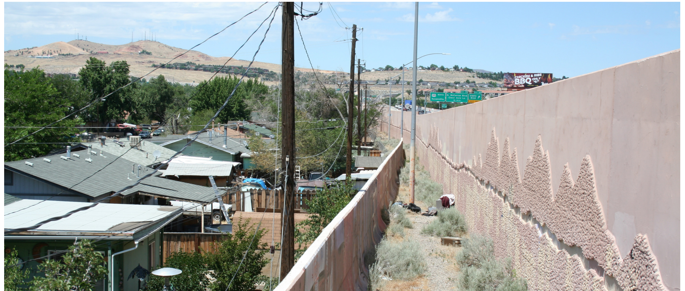
The view north along US 395 and Butler Street, just north of the Spaghetti Bowl. The taller wall on the right is a traffic noise barrier, and the shorter wall on the left is a retaining wall.
