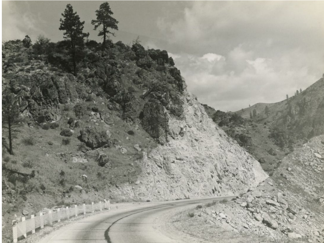
Figure 24. Image of rock cut one-quarter mile east of the California state line. 137
