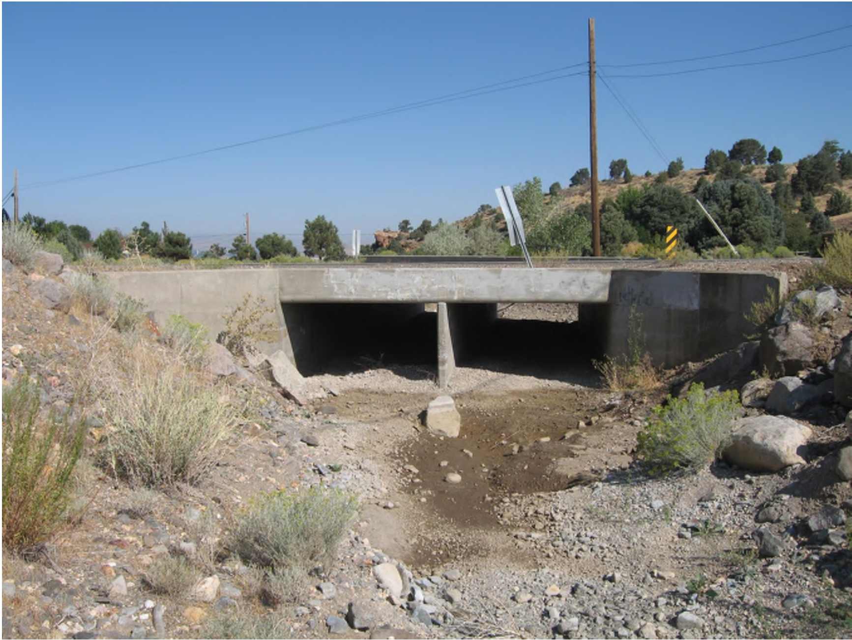
Photo: Bailey Canyon Creek Culvert Crossing at Toll Road. Looking downstream (northwest) at 2-8'x5' Concrete Box Culverts. (Photo Date: 9/16/2011)
