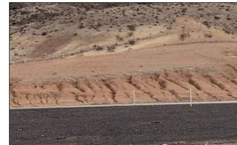
Erosion along northbound I-15 cutslope
