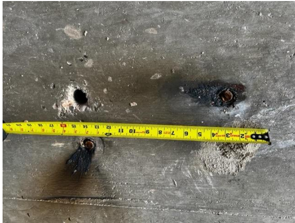
3.1 (2" dia. drill hole w/ exposed re-bar x3)
