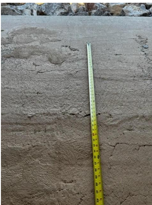
4'x4' delaminated floor west end of cell 2
