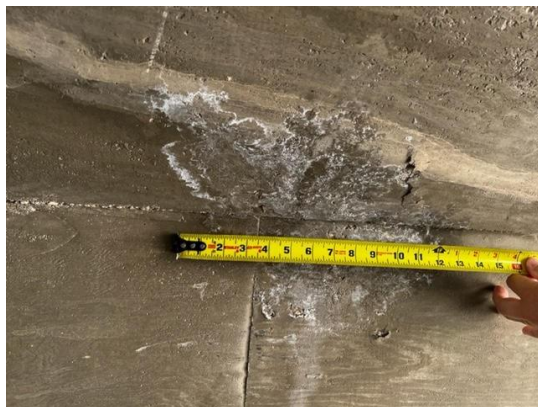
1.3 (Shrinkage cracks less than 1/64")
