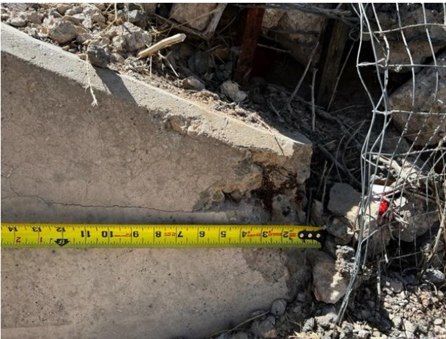
1.1 (6" x 6" Spall concrete)
