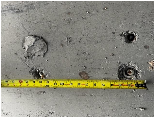
2.1 (2" dia. drill hole w/ exposed re-bar x 3)
