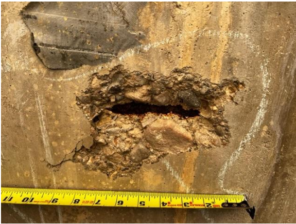
2.1 (9" x 5" spall and corroded rebar)
