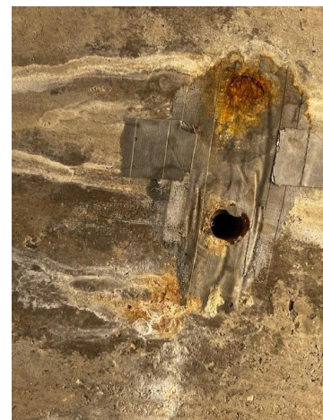
3.2 (2" dia. drill hole and corroding rebar through patch work)
