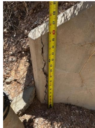
4.1 (16" spall -NW Wingwall)
