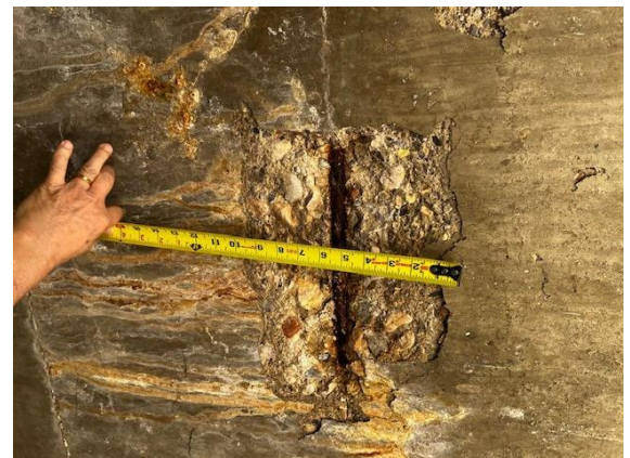
1.4 (10" x 16" spall and corroded rebar)
