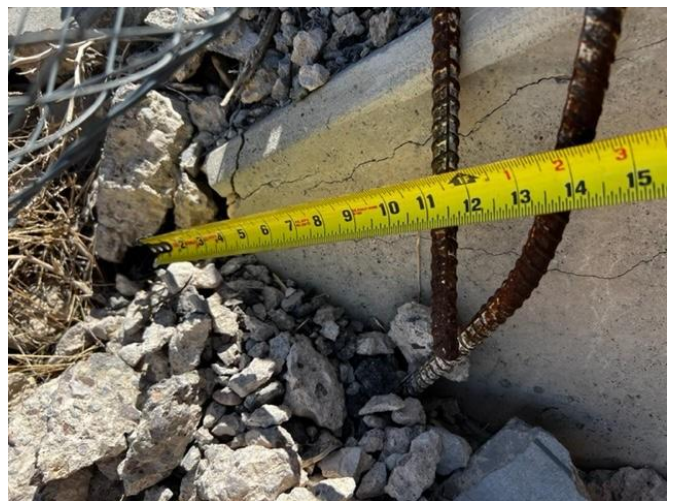
4.1 (15" spall at wing wall corner)
