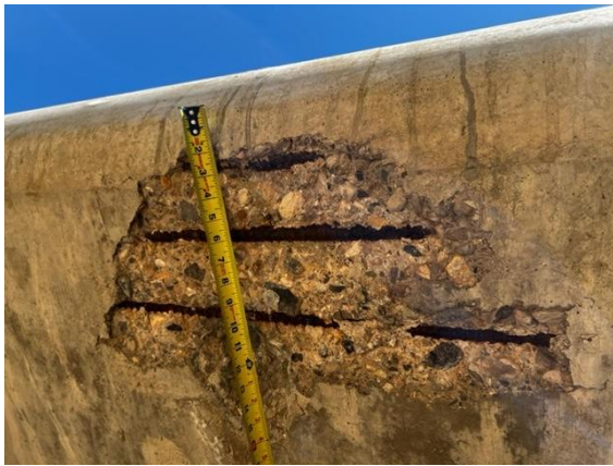
3.3 (1'x 2' spall with exposed re-bar)
