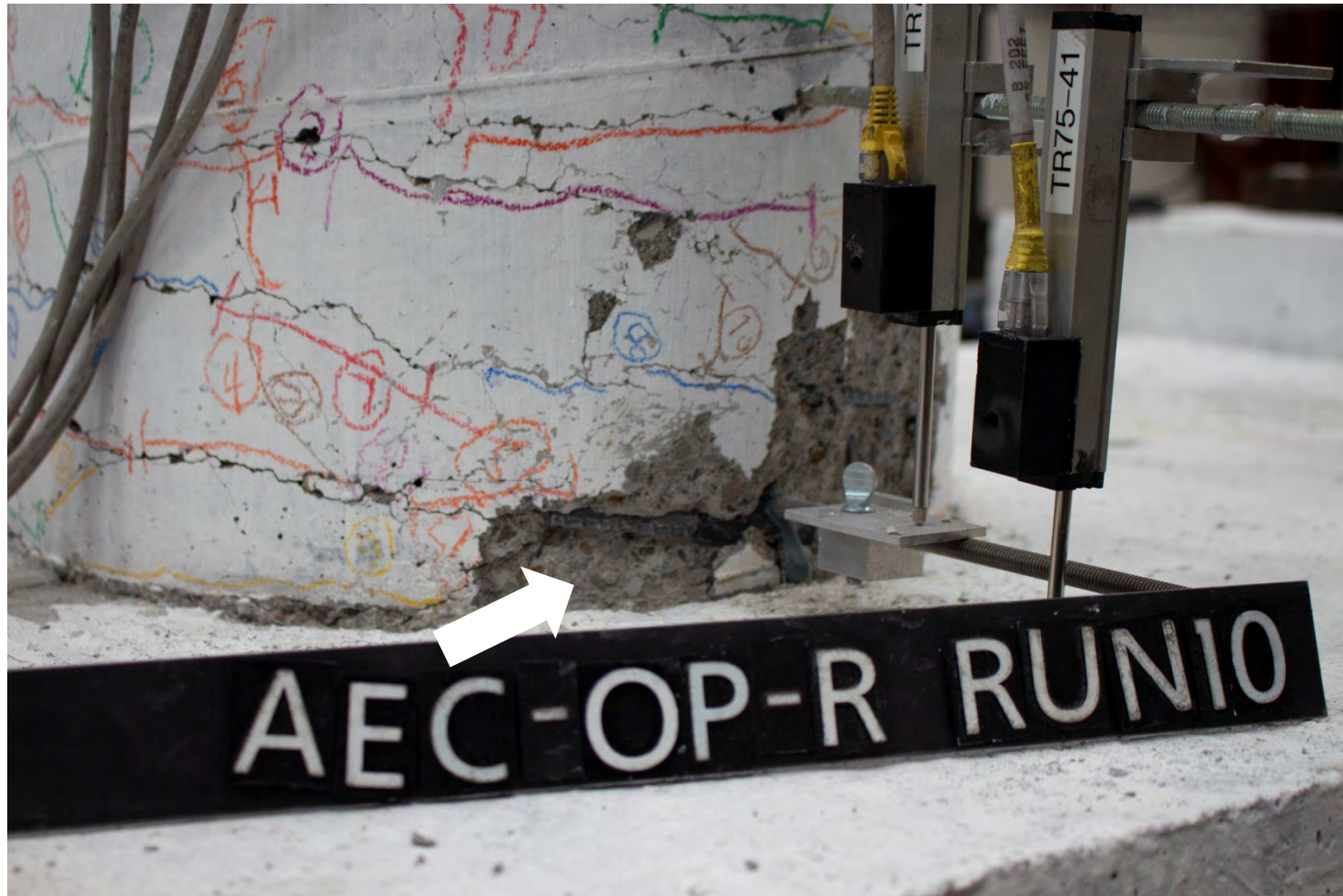
Figure 3.13 Concrete spalling in the north direction (run #10)
