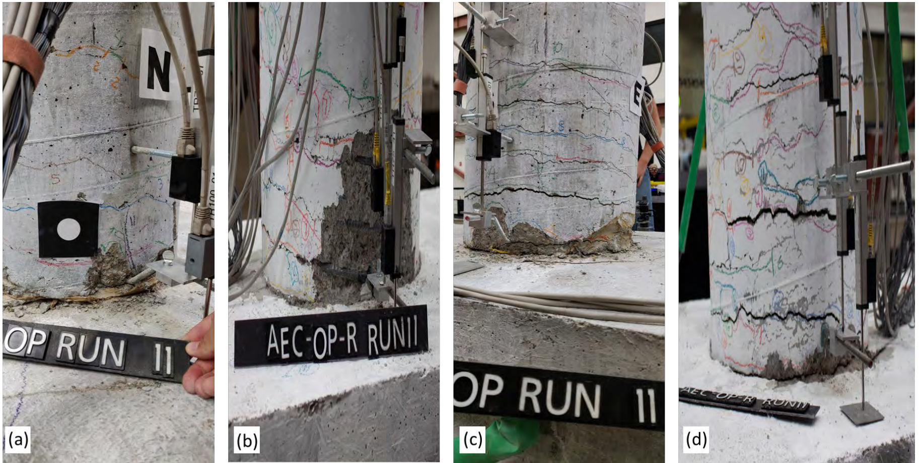
Figure 4.3 Comparison of concrete spalling as observed from the specimens tests located at: (a) north section of the original specimen, (b) north section of the repaired specimen, (c) south section of the original specimen, and (d) south section of the repaired specimen
