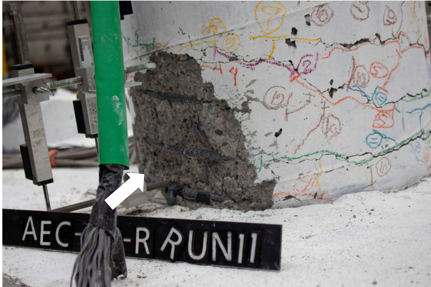
Figure 3.14 Concrete spalling in the north direction (run #11)
