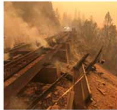
A damaged ridge on BNSF railroad in Northern California. Source: BNSF
