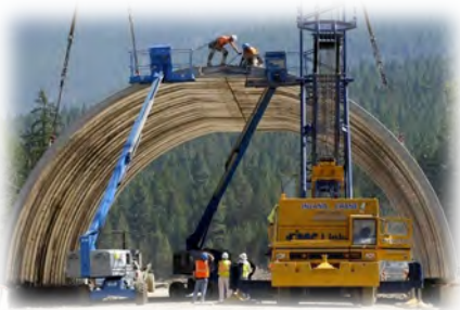
Figure 5. Constructing large structures such as this wildlife overpass entail inclusion of these structures in early planning, such as in the long-range plans of agencies. Photo Credit: T. Brennan.
