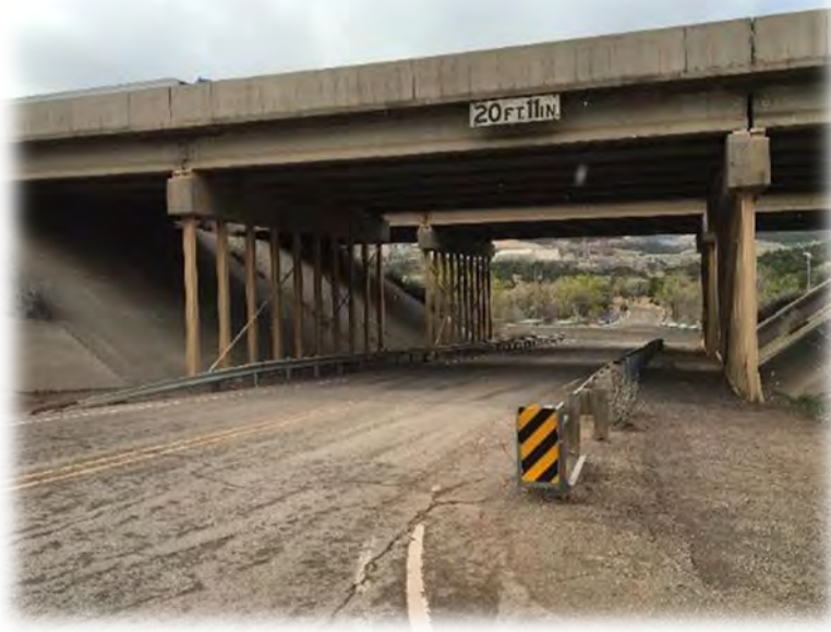
Figure D-3. New Mexico Tijeras Canyon retrofit of Public School interchange under Interstate 40 with a natural substrate path to the side of the paved surface to facilitate wildlife movement beneath the highway bridge. There are no known successful passages by wildlife. Photo Credit: J. Gagnon, Arizona Game and Fish Department.
