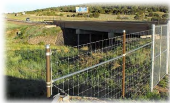
Figure D-1. Bridge under Interstate 40 in New Mexico, with wildlife exclusion fence placed to guide wildlife to the existing bridge. Photo Credit: J. Hirsch and M. Watson.
