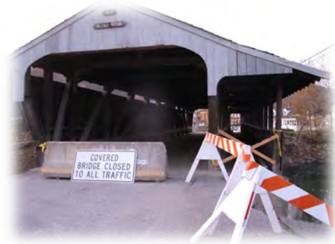
Figure 2-5. A covered bridge in Vermont was almost washed away from the river surge due to Hurricane Irene in 2011. Photo Credit: P. Cramer.
