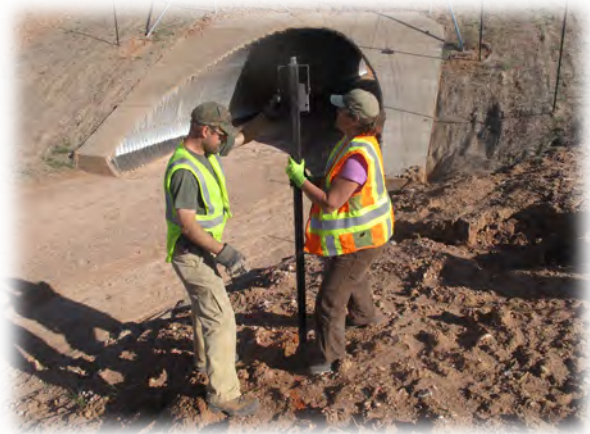
Figure E-4. Wildlife researchers place a monitoring camera at the entrance to a wildlife crossing structure in Utah along US 89. Photo Credit: J. Gagnon.
