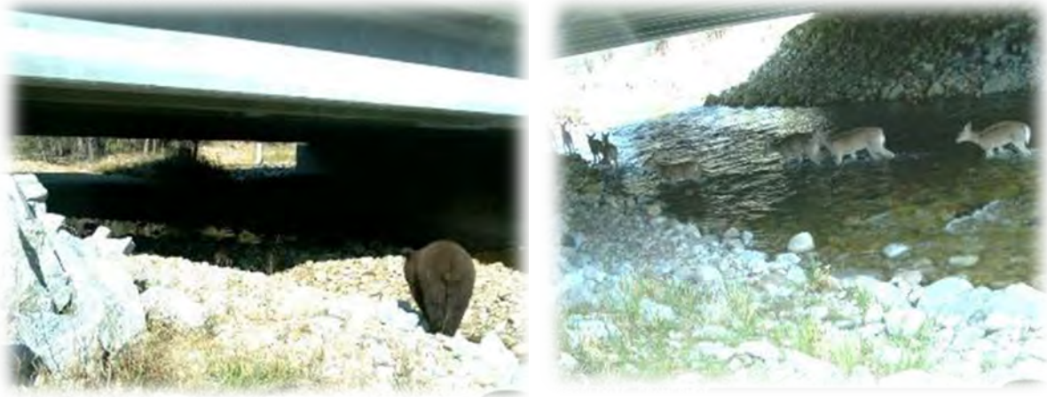
Figure D-16. In Montana, black bear and white-tailed deer used bridged wildlife crossing structures with water features. Photo Credit: P. Cramer and Montana Department of Transportation.
