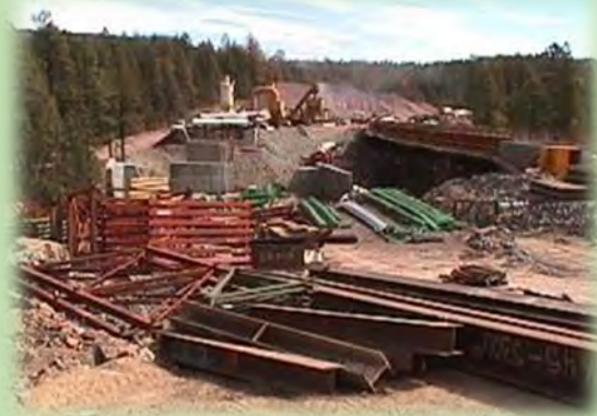
Figure A-17. Contractor use area, Arizona's State Road 260, on the Tonto National Forest. Photo Credit: T. Brennan.
