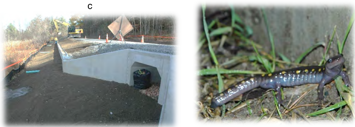
Figure 3-31. Vermont Transportation Agency built an amphibian wall and crossing structure with a natural substrate to facilitate spotted salamander movement to breeding ponds. There were also native plants planted at both ends. Photo Credit: Vermont Transportation Department, and C. Slesar.
