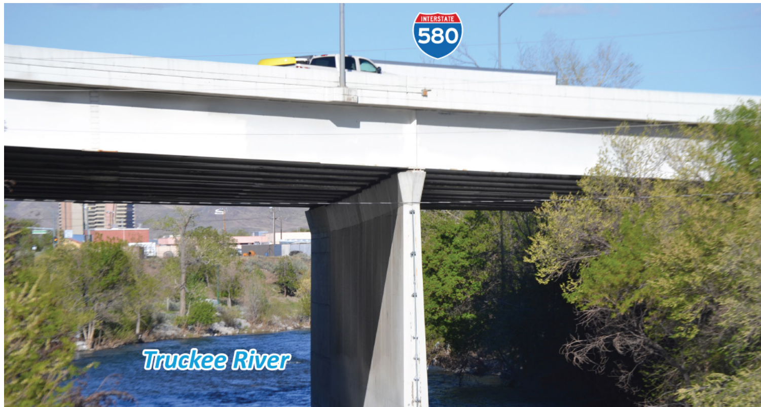
I-580 bridge over the Truckee River, and the bridge pier supporting it.
