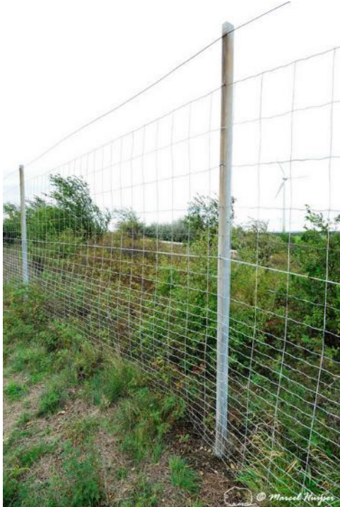
Figure 68. Mesh wire wildlife fence with metal poles on top of multifunctional overpass (wildlife, bicyclists, pedestrians; about 100 m wide), across A4 motorway, Parndorf, Austria. The overpass is designed for farmers, agricultural machinery, hunters and wildlife including roe deer ( Capreolus capreolus ) and European hare ( Lepus europaeus ). Mesh size is small towards the bottom.
