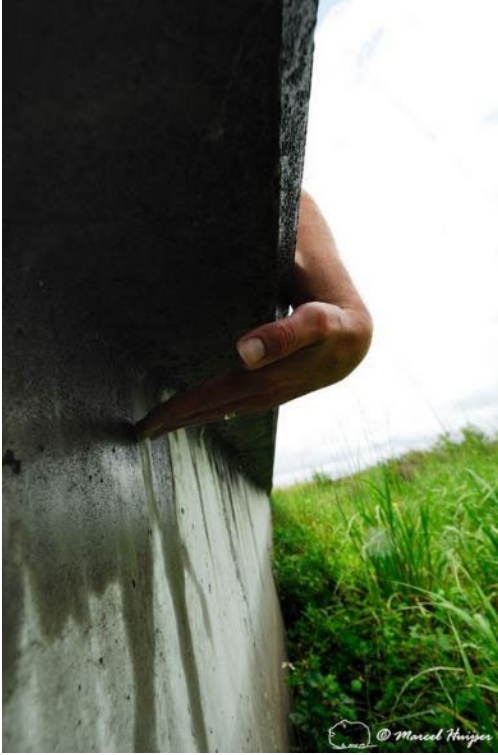
Figure 72. Barrier wall integrated into the roadbed with overhang for reptiles, amphibians and small mammals, U.S. 441, Paynes Prairie Ecopassage, south of Gainesville, Florida, USA.
