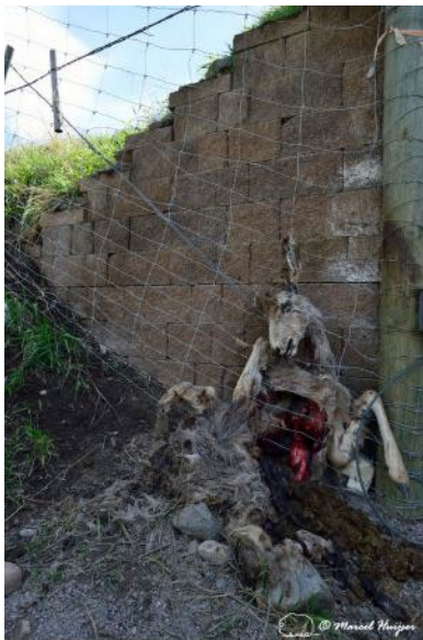
Figure 53. Mule deer ( Odocoileus hemionus ) got stuck between wildlife fence and the wing wall associated with a wildlife underpass and dies, Montana, USA. The fence should be snug up to the wing wall. Here the last fence post was close enough to the wing wall but the second to last post allowed for a funnel like configuration making the deer believe it could potentially pass in between the wall and the fence. When it realized it could not go forward anymore it tried to turn itself around and then got stuck and died. It is important that both the post and the fence are positioned such that no space is left between the wing wall and the fence.
