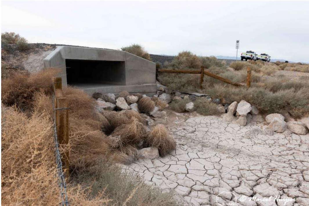
Figure 112. A culvert with a heavily eroded outflow near Indian Springs, Nevada, USA. Inaccessible to desert tortoises.
