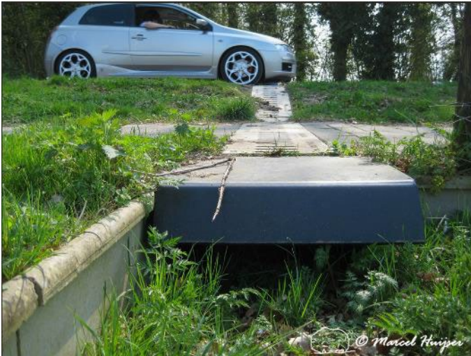
Figure 88. Cover close to the entrance of an amphibian tunnel, The Netherlands.
