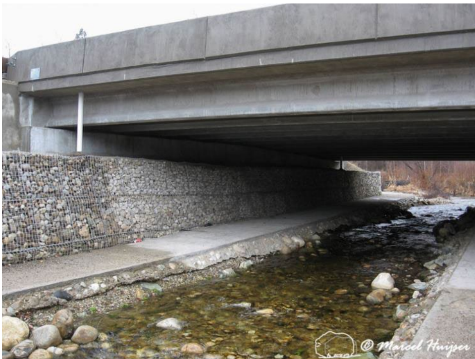
Figure 23. Pathway for large mammals in an underpass (bridge) primarily designed for water (stream), US Hwy 93 S, Bitterroot Valley, Montana, USA.
