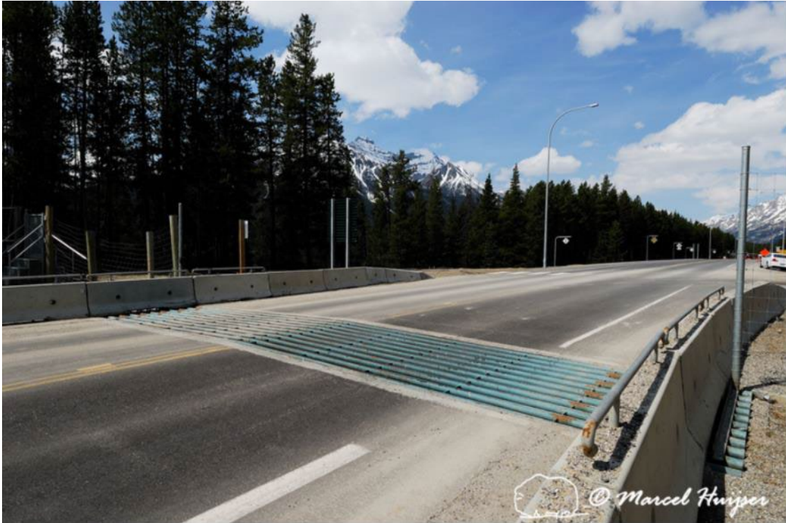
Figure 27. Fence-end brought close to the edge of the pavement, protected by Jersey barriers. Also note that there is a wildlife guard embedded in the travel lanes, Alberta, Canada.
