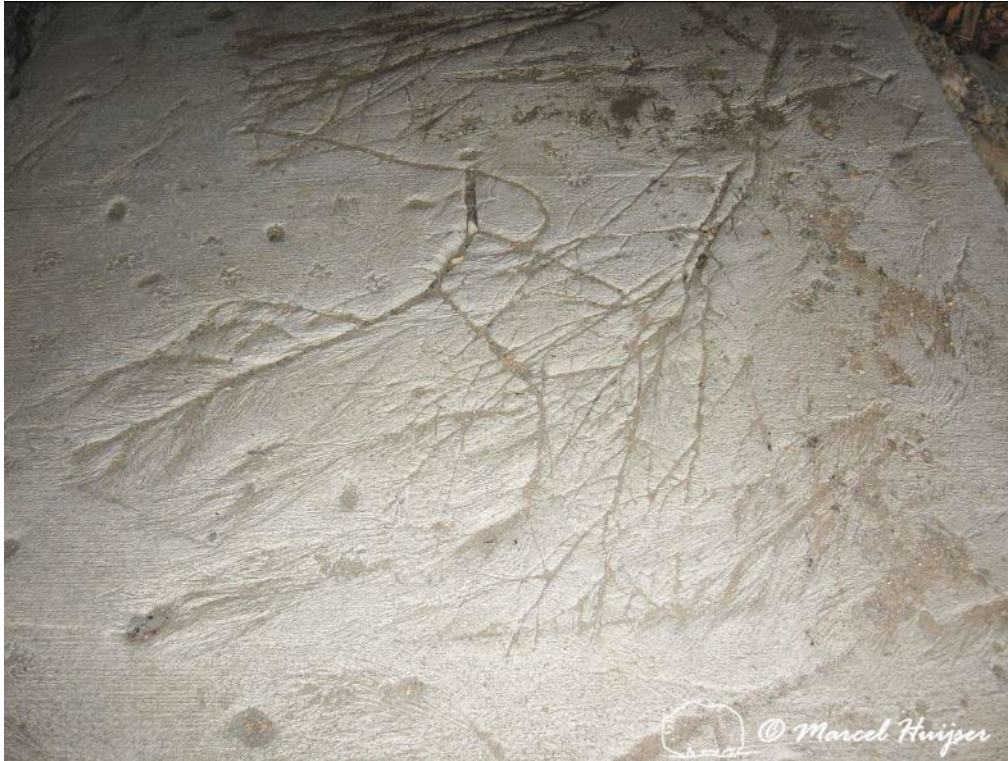
Figure 94. Imprints in concrete surface in wildlife underpass to make it less slippery for wildlife, US Hwy 93 S, Bitterroot Valley, Montana, USA.
