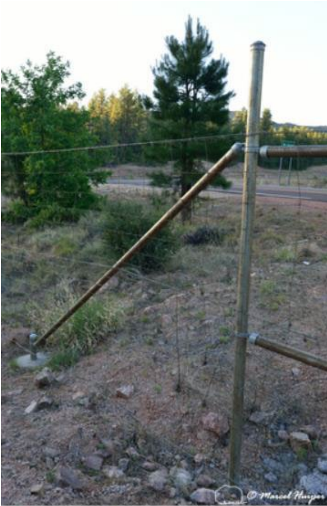
Figure 13. Wildlife fence with metal posts as a barrier for deer ( Odocoileus spp.) and elk ( Cervus canadensis ) along SR 260, east of Payson, Arizona, USA. Some of the metal posts are set in concrete.
