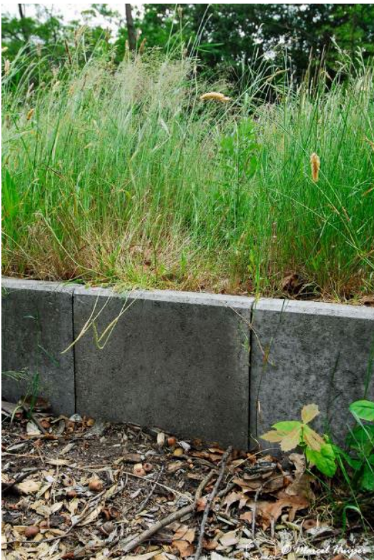
Figure 66. A “barrier wall” (concrete) integrated into the roadbed for common toads ( Bufo bufo ), Deelenseweg, between Hoenderloo and Arnhem, Gelderland, The Netherlands.
