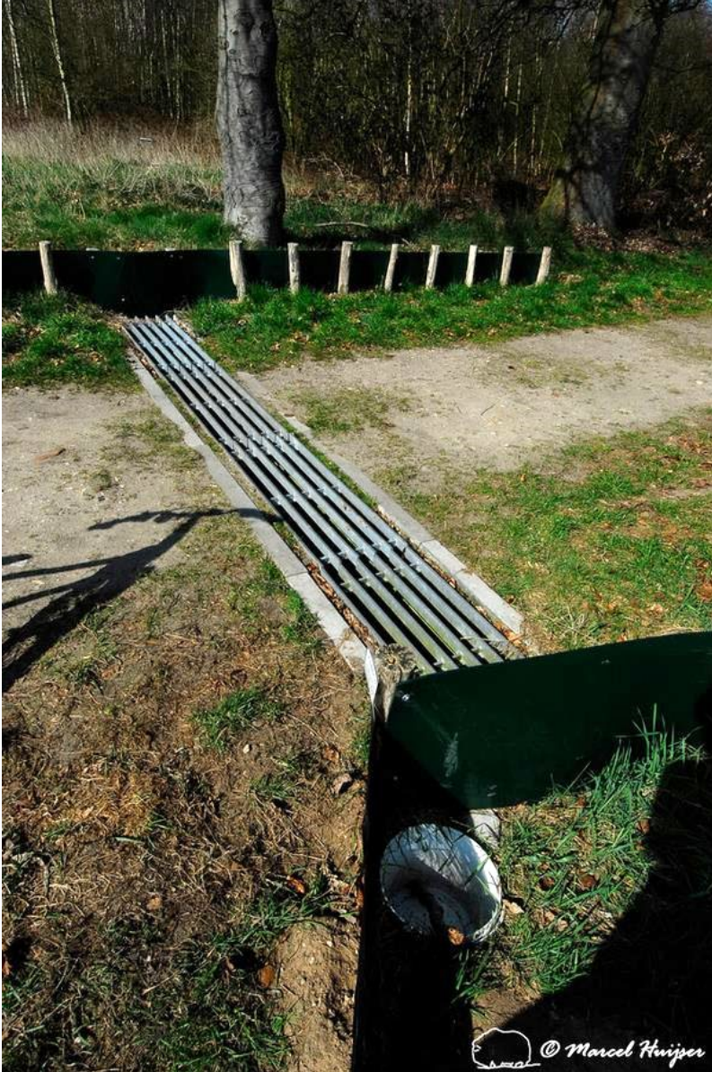
Figure 75. ABS plastic sheets to keep common toads off the highway (highway is to the left of the image), and an amphibian tunnel under an access road. Amphibians that approach the access road would fall in between the bars. Amphibians that travel along the barrier would go through the tunnel, continue to travel along the barrier on the other side of the access road until they encounter a tunnel that allows them to cross to the other side of the highway.
