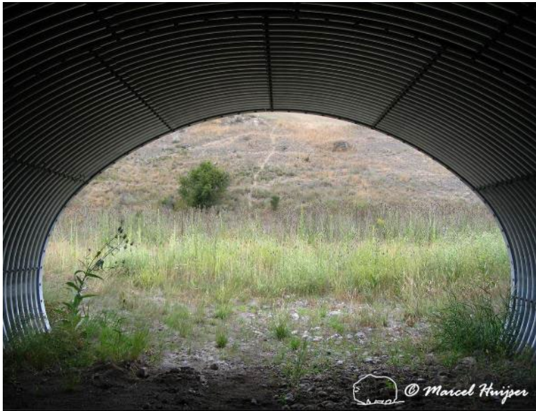
Figure 82. Corrugated metal culvert with bottom placed below the ground level of the surroundings, US Hwy 93, near Ravalli, Flathead Indian Reservation, Montana, USA.
