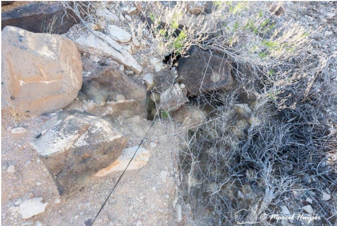
Figure 111. A culvert blocked by rocks under the road to the overlook, Childs Mountain, Cabeza Prieta National Wildlife Refuge, Arizona, USA.
