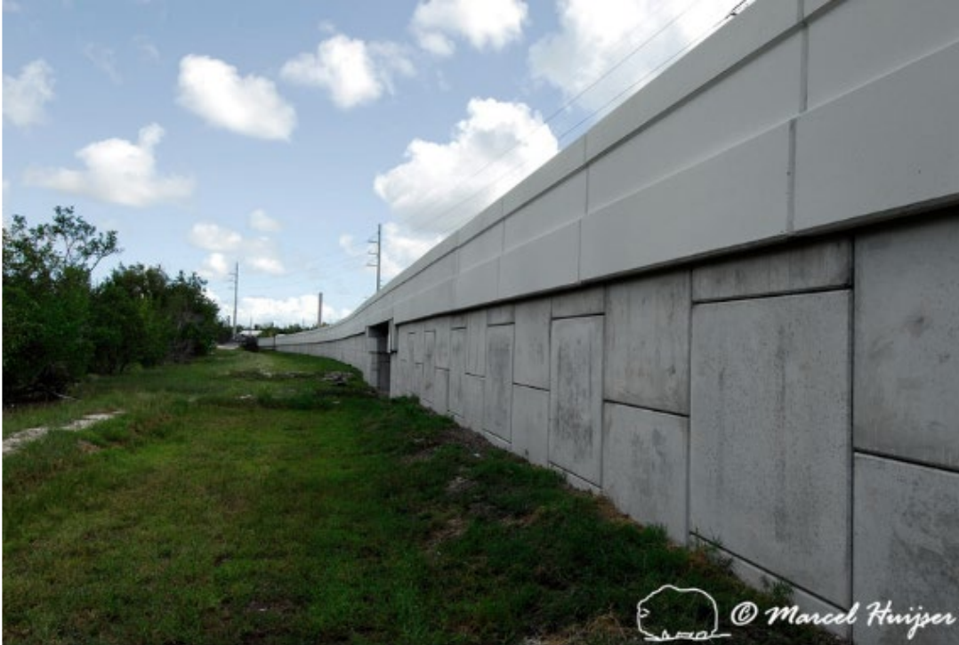
Figure 6. A barrier wall because of raised roadbed for wildlife underpass for Key deer (8 m wide, 3 m high), US Hwy 1, Big Pine Key, Florida, USA. A barrier wall can be considered if concerns for landscape aesthetics do not allow for a fence.
