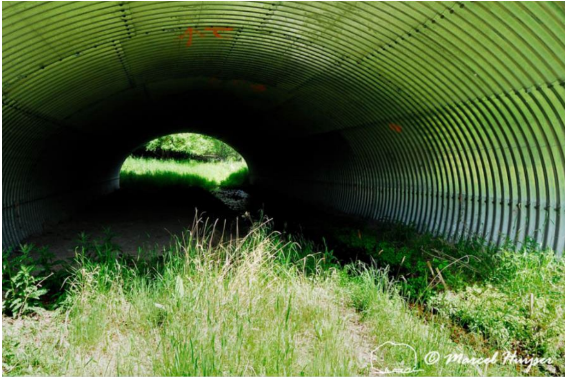
Figure 25. Multi-functional underpass for wildlife and water with soil and rocks that cover the bottom of the culvert, US Hwy 93, near St Ignatius, Flathead Indian Reservation, Montana, USA.
