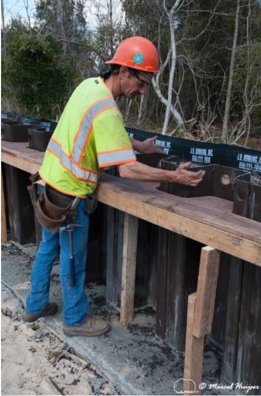
Figure 65. Barrier wall for turtles, alligators, snakes and amphibians, Lake Jackson Ecopassage, Tallahassee, Florida, USA. The barrier wall was under construction when the image was made.
