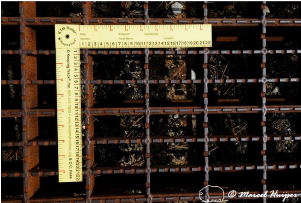
Figure 39. Detail of the modified bridge grate material used for wildlife guards installed at access roads along US Hwy 93, near Ravalli, Montana, USA. This material is more suitable for pedestrians and cyclists compared to the bars of a traditional wildlife guard or cattle guard.
