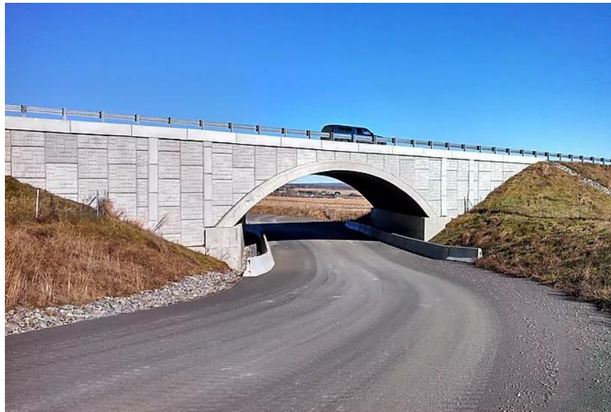
Figure 16: CFFT bridge built by AIT in Augusta, Maine. The bridge uses 22, 15in diameter carbon-fiber tubes to make a span of 54ft, is 55ft wide, and has a rise of 12ft above the concrete abutments to allow enough clearance for traffic once they are placed on the pre-cast concrete foundation.
