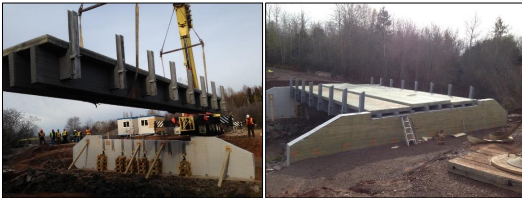
Figure 12: Example of FRP bridge made by Guardian Bridge Rapid Construction for a two lane road over a creek, the bridge spans 15m; (Left) a triple-tee span being placed by a crane, (Right) all three spans placed on top of an FRP abutment.
