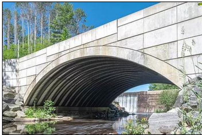
Figure 9: The Perkins Bridge in Belfast, Maine, made with a CFFT and FRP panels. The bridge spans 47ft 7 inches (in), has an 11ft rise, and is 45ft wide. It is made with 16, 15in diameter tubes. Each arch weighed 250 pounds (lbs) before they were filled with concrete [61].
