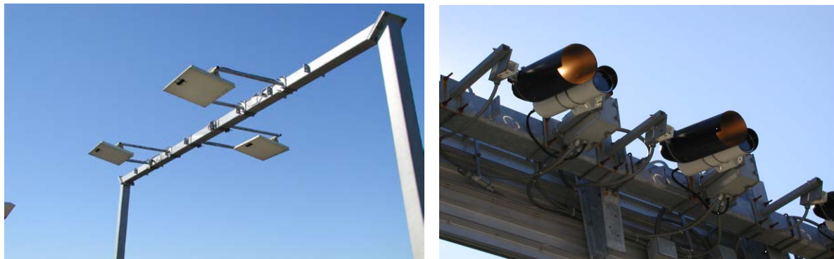
Figure 1-7: Cameras and Overhead RF Antenna
