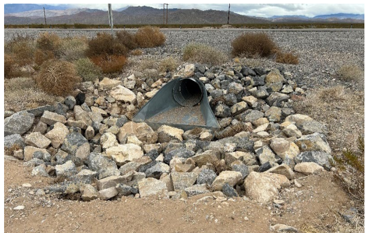
Photograph 2: Example of corrugated metal pipe (CMP) with voids in large rock riprap.
