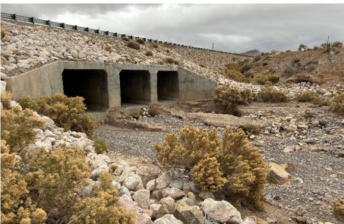
Photograph 1: Example of 3-cell reinforced concrete box (RCB) culvert with headcut along SR 160.
