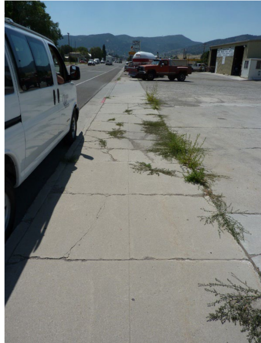
Sidewalks along US-50 and US-93 are deficient and aged.
