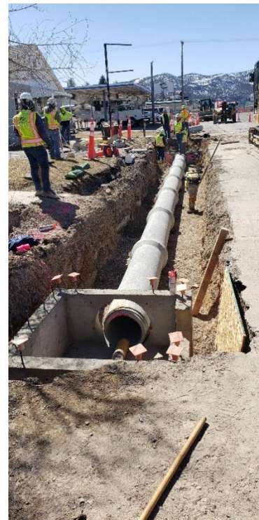
Storm drainage and water and sewer facilities will be upgraded to match those completed in Phase 1.
