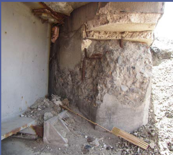
Example of concrete spalling.
