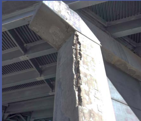
Example of concrete spalling.
