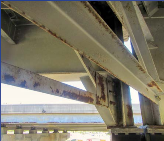
Example of steel girder corrosion along bridge.
