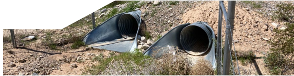
Dual-purpose drainage structure and tortoise crossing, with tortoise fencing along US 93.
