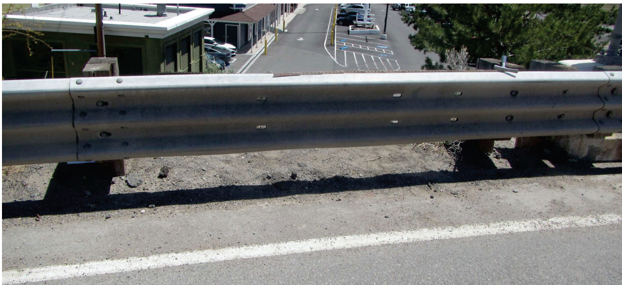
Missing posts on approach rail transition can lead to barrier failure in case of a traffic incident.
