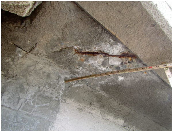
Spalled concrete with corroded rebar in the deck overhang (I-774E bridge)
