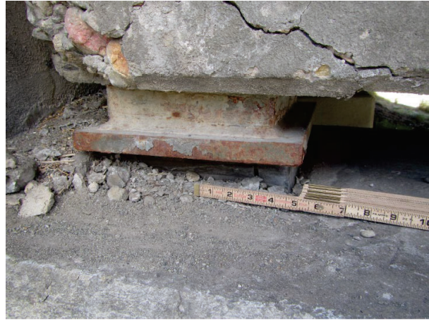
Distressed bearings (I-774W bridge)
