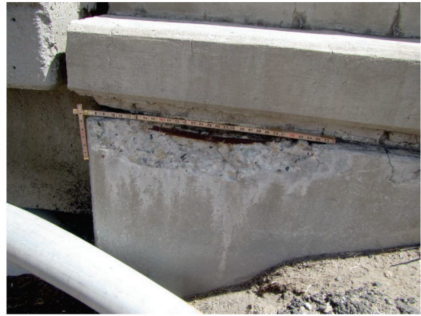
Spalled concrete (I-774W bridge)
