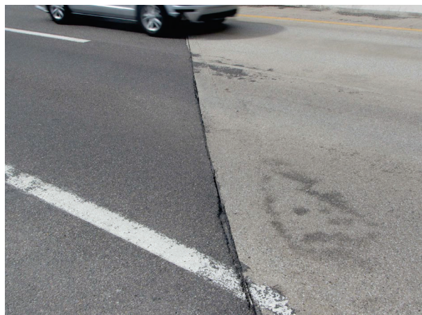
Failure of relief joint.
