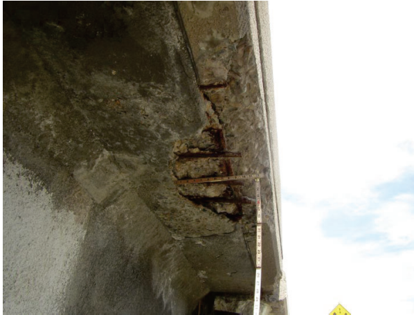
Spalled concrete with corroded rebar in the deck opening overhang (I-774E bridge)
