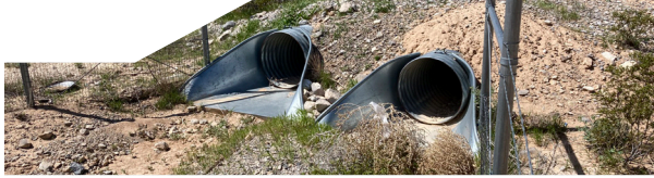
Dual-purpose drainage structure and tortoise crossing, with tortoise fencing along US 93.
