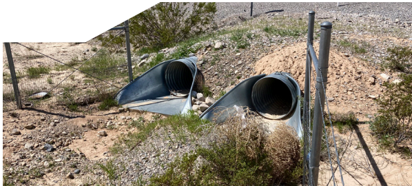
Dual-purpose drainage structure and tortoise crossing, with tortoise fencing along US 93.
