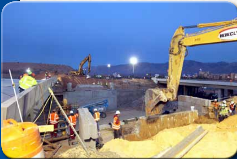
Work being performed on the new bridges at the West Mesquite Interchange.
