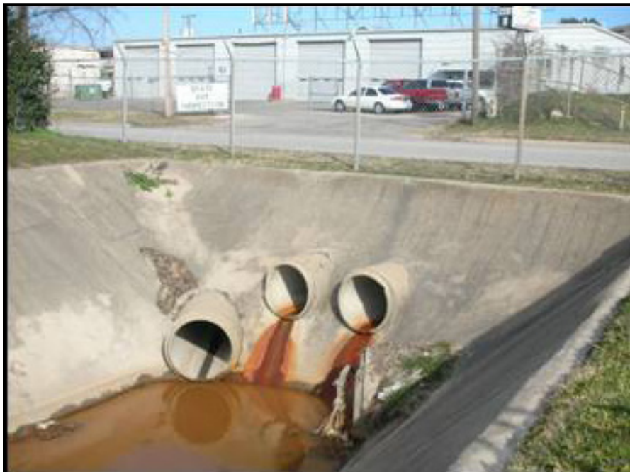
Figure 1-35. Obvious staining can be seen at two of the three outfalls. The rust red color indicates iron staining and may be due to an illicit discharge. (Photo from the City of Fort Worth, Texas)
