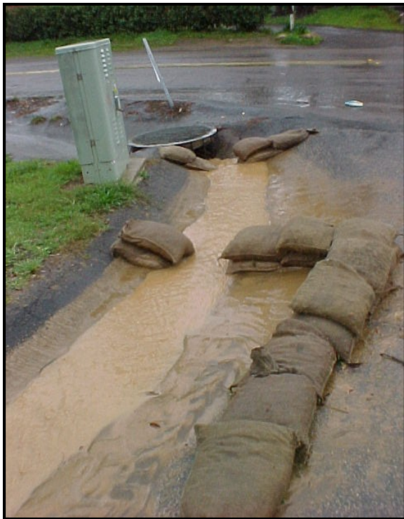
Figure 1-21. Highly turbid water from a construction site flowing into the MS4. Note that the inlet protection bags have been pulled to prevent flooding – an approved practice during high volume runoff events (Photo from NDEP)
