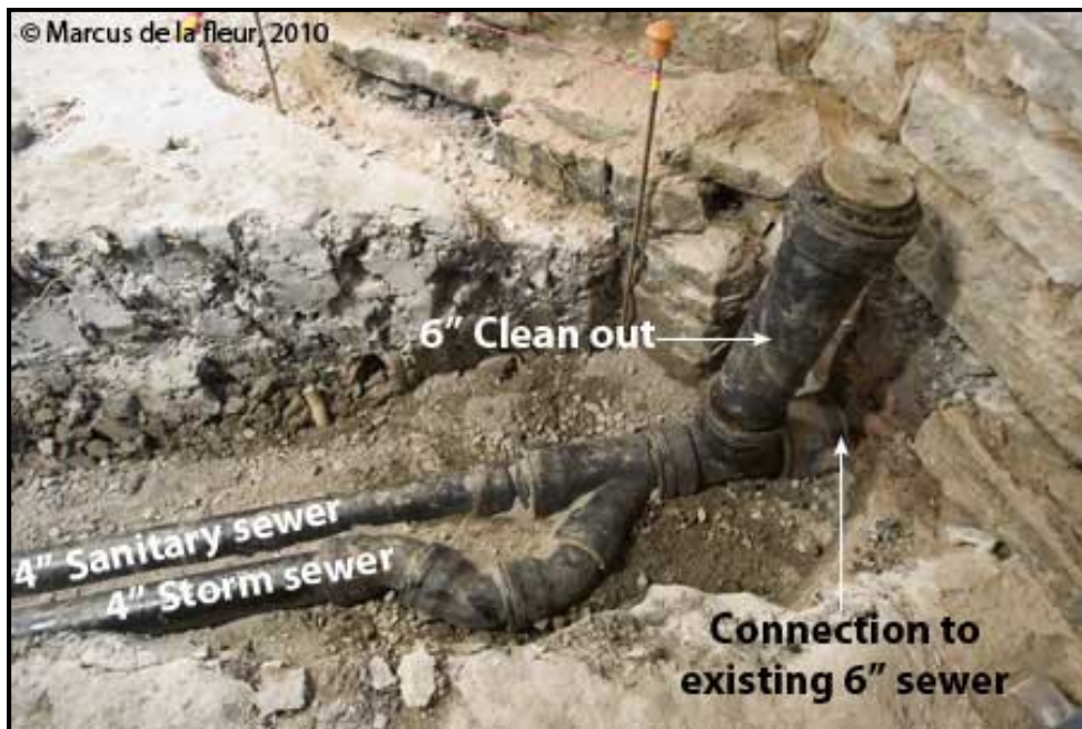
Figure 1-2. The mode of entry to the MS4 is a “direct” connection of a sanitary sewer line to a storm drain pipe. The flow of sewage into the storm drain was “continuous” in nature since the sewer flowed uninterrupted. (Photo from Marcus de la fleur)
