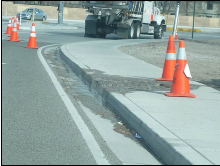
Figure 1-5. A sanitary sewer is surcharging (overflowing) raw sewage as a result of a plugged sewer line. The sewage then flows into the gutter and into a drop inlet. In some cases, if it is not disrupting service, it can be some time before a situation like this is recognized and mitigated. This is an “ indirect ” mode of entry that is most likely a “ transient ” or “ intermittent ” discharge situation. In some cases, sewer overflows can be overlooked for long periods resulting in a “ continuous ” discharge. (Photo from the City of Reno)
