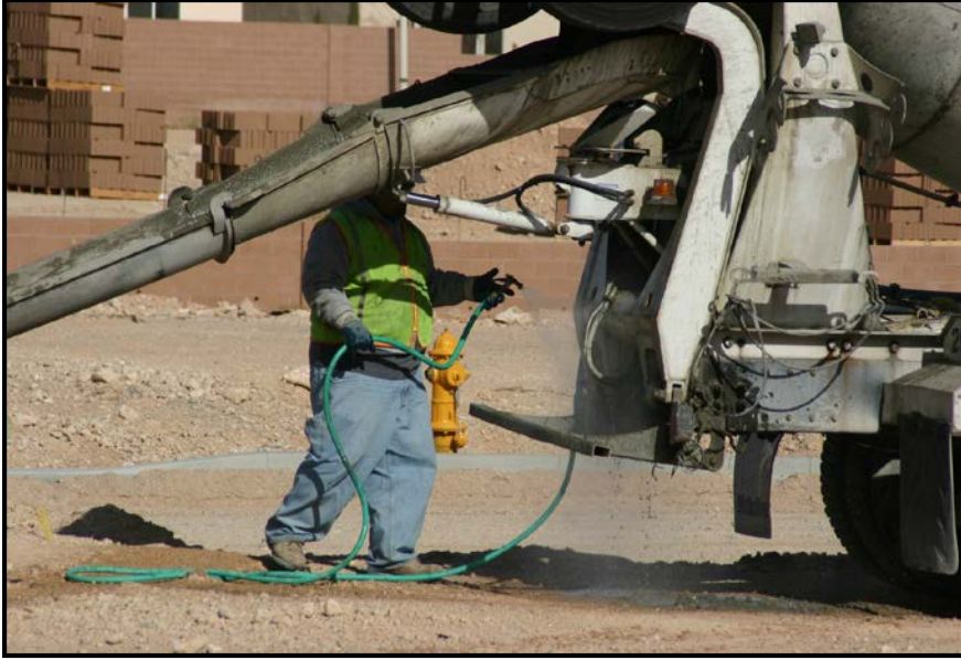
Figure 1-7. In this situation, a concrete truck is washed onto the ground and not into an approved washout facility. If this material was washed into the MS4, this would be considered an “indirect” mode of entry and “transient” in frequency. (Photo from NDEP)
