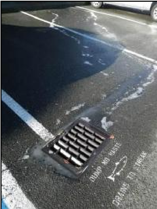
Figure 1-27. The foam on the parking lot shown here was from car washing activities at a car sales lot. While individual, residential car washing is permissible, commercial car washing is not. (Photo from the Washington State Department of Transportation)
