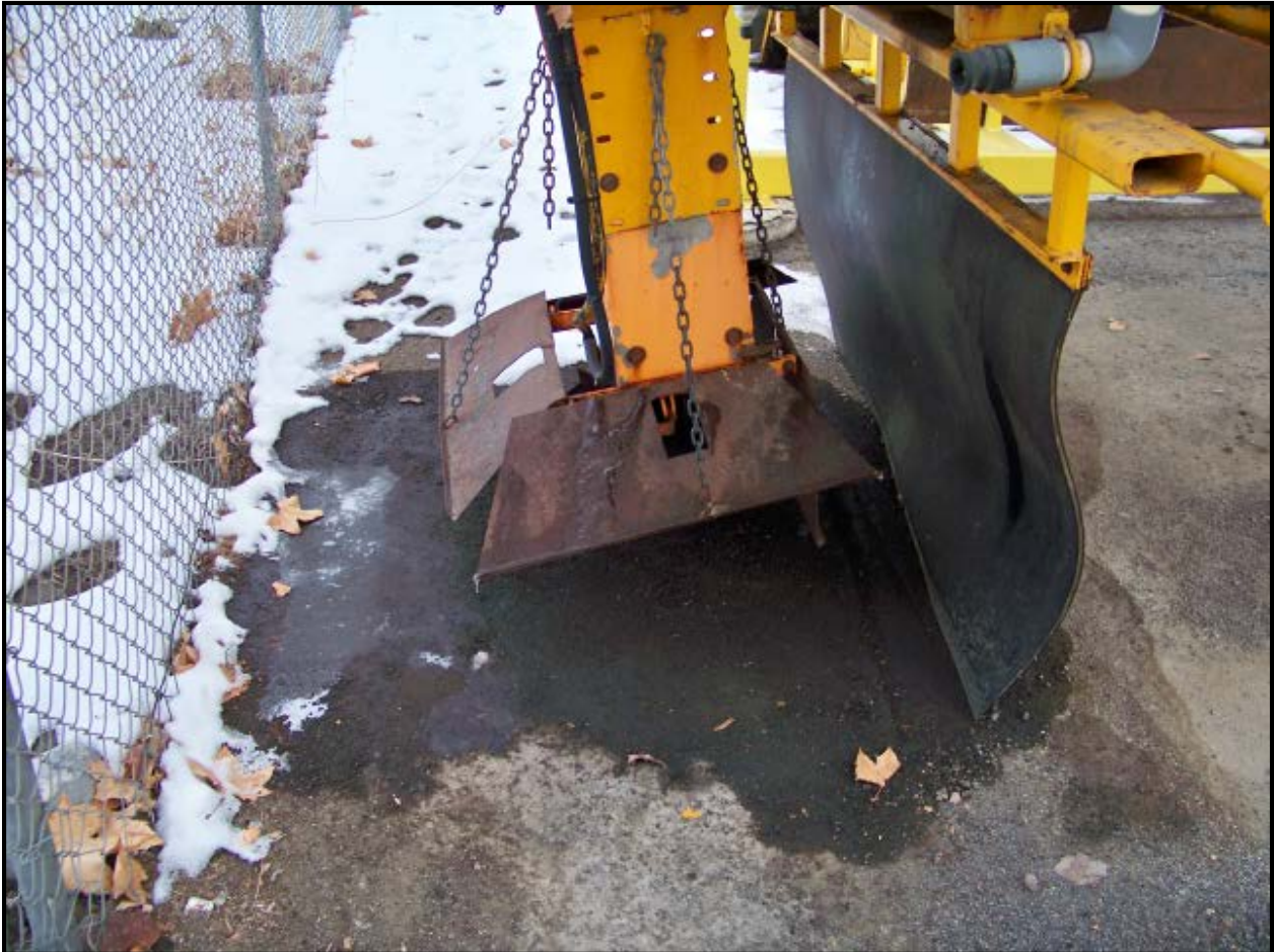
Figure 1-33. While no active leaks are occurring, evidence of past hydraulic fluid discharges are evident. (Photo by Stantec)
