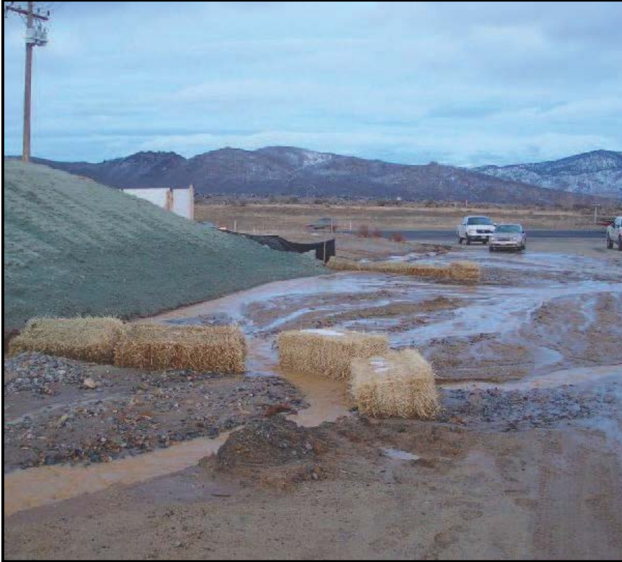
Figure 1-22. This photo shows failed BMPs at a construction site and highly turbid stormwater runoff. (Photo from NDEP)
