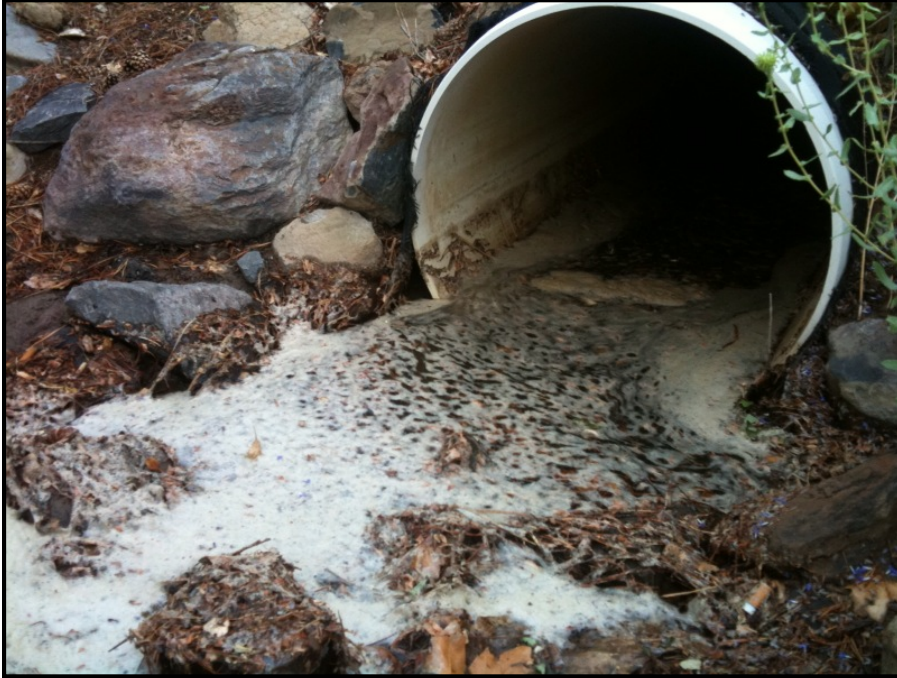
Figure 1-28. This photo was taken right after a heavy summer thunderstorm at a small neighborhood park. The foam here was caused naturally from decaying organic matter. (Photo by Stantec)
