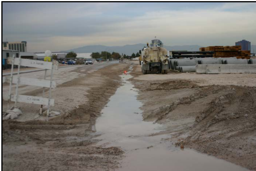
Figure 1-6. In this situation, sediments were discharged from a construction site and flowed into the storm drain inlet with no BMPs in place. This is regarded as an “ indirect ” mode of entry and would be considered “ transient ”. (Photo from NDEP)
