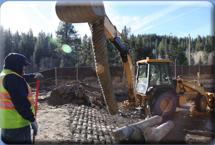
Spoooner Decant Facility
