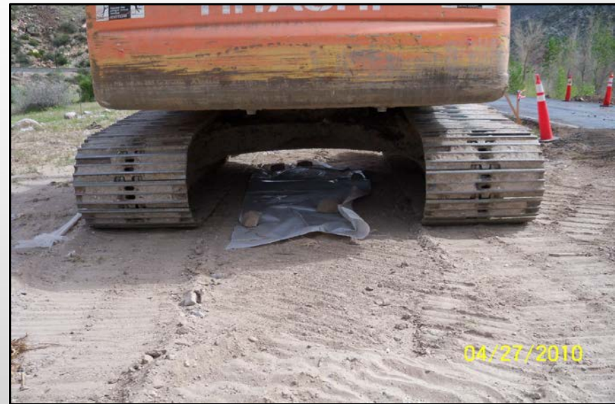
EQUIPMENT LEAK MANAGEMENT
