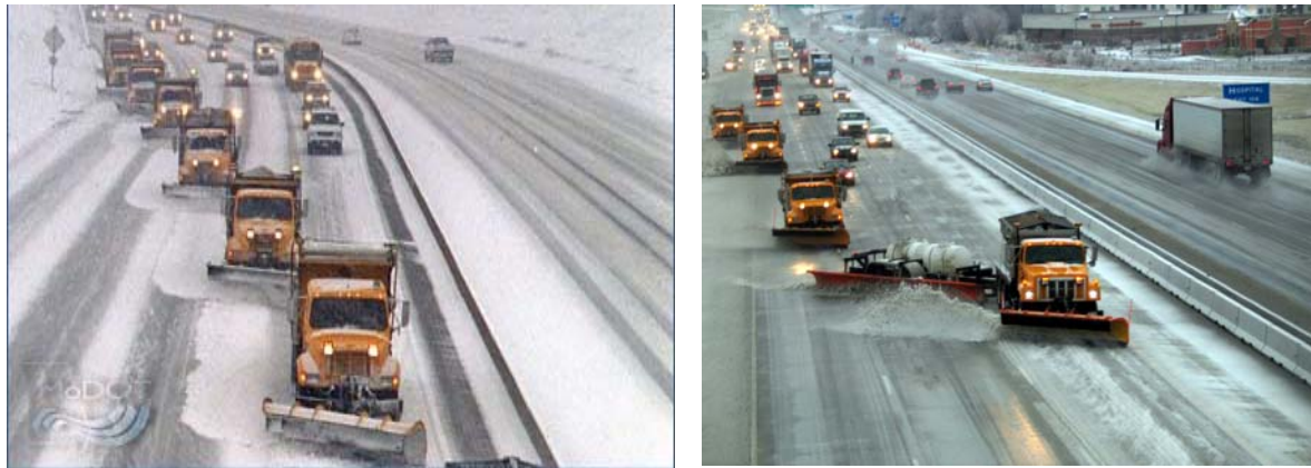
Figure A.6 Missouri Gang Plowing with and without Towplow plowing 28' of Pavement
