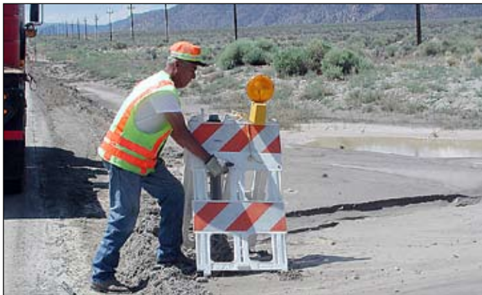
WARNING—With shoulders nothing more than treacherous mud on SR-359, Juan Lopez sets out a warning to motorists to stay on the pavement.
