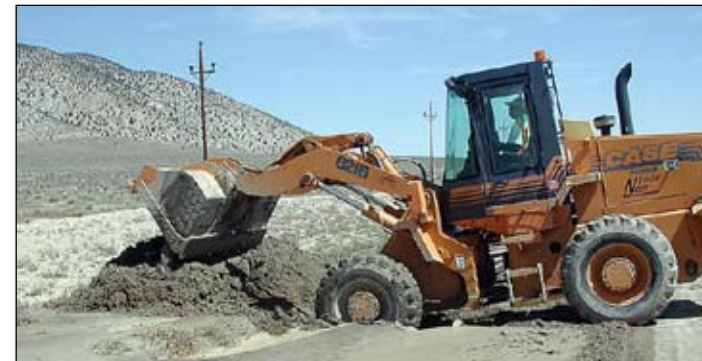
DEFT TOUCH—Charles Jones guides a loader with a sure hand on SR-359, moving mud from the shoulder and changing the landscape around a culvert. Jones also took material from the high side of the road to build up the shoulder on the low side.
