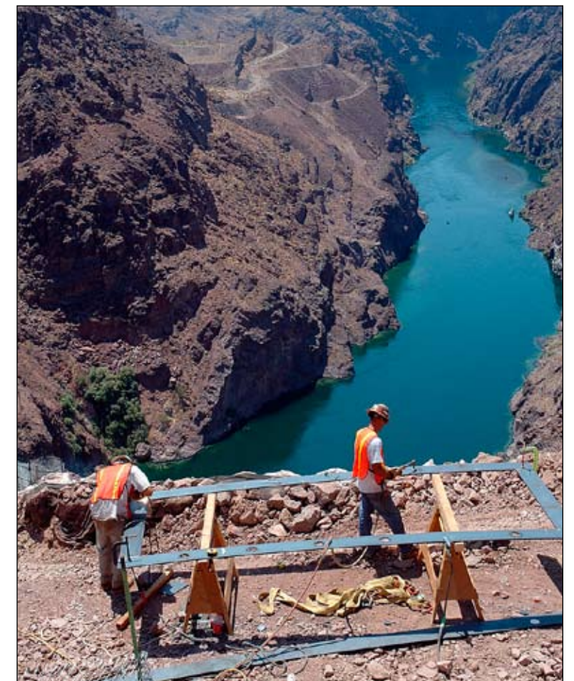
Near the Hoover Dam, the Mike O'Callaghan-Pat Tillman Memorial Bridge is being built to span the Colorado River.
