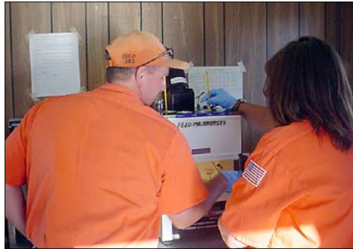
Roger Weber (left) and Janet Van Camp are the Ely team members who helped test materials for the Pioche-area chip seal job.
