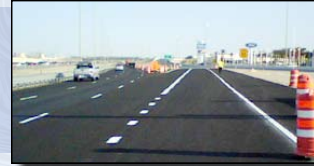
Widened new blacktop near Ann Road is just one benefit of NDOT's recent U.S. 95 restriping project.
